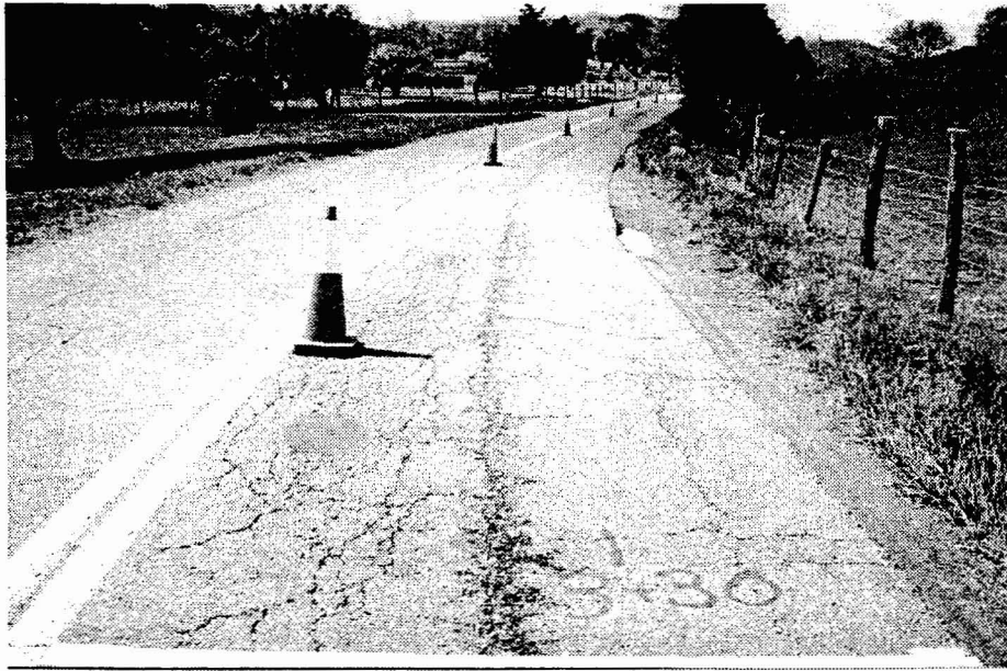
Photo 15. Severe Fatigue Damage with Patched Pothole at Site 1: Route 607, Wythe County, April 2000
