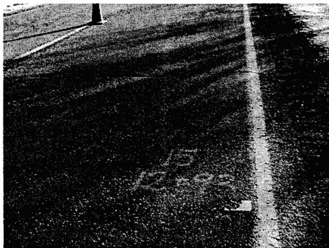
Photo 3. Photographic Documentation of Site 15. Note the segment's unique identification number and the transverse crack.
