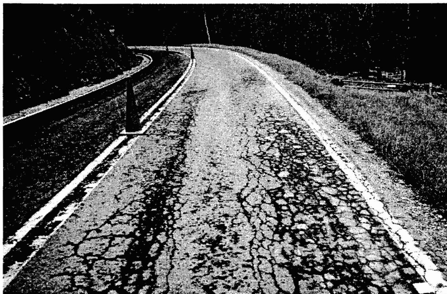
Photo 16. Severe Fatigue Damage at Site 9: Route 93, Grayson County, April 2000
