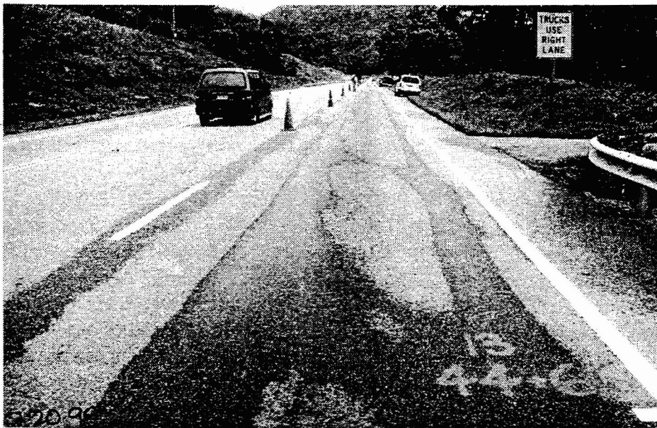
Photo 18. Wheel Path Rutting at Site 13: Route 58, Lee County, July 1999. Note standing water in wheel paths.
