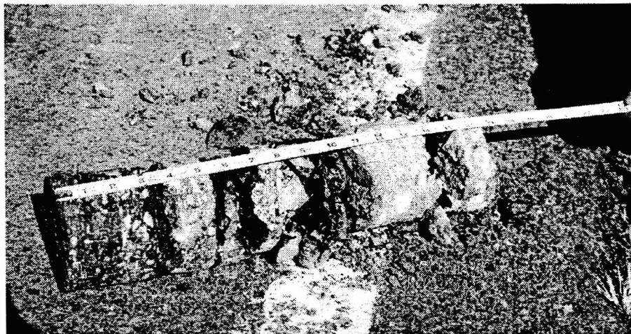
Photo 9. Extracted Core. Note the deterioration of asphalt at 7 to 10 inches.
