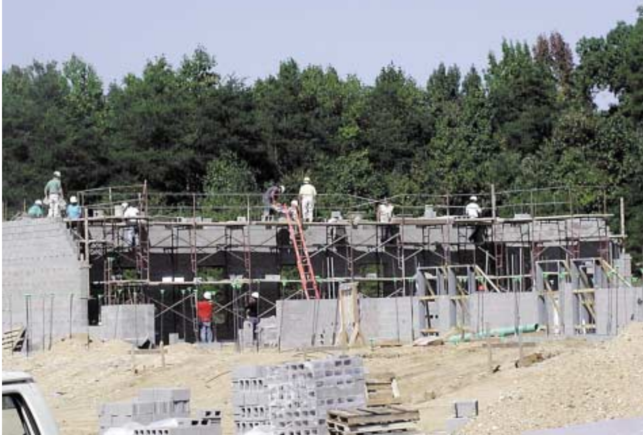
Construction site of Danville Community College's new Regional Center for Advanced Technology at the Danville Cyberpark. Projected occupancy - June 2005.
