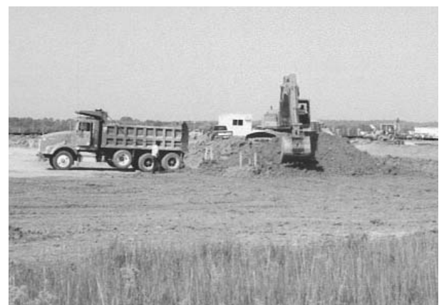
The Airports RLF loaned the City of Manassas $1,401,714 for the construction of pad sites, an access road, and utilities to support four new corporate hangar facilities. The City will save $100,143 in interest costs over the life of the loan.
