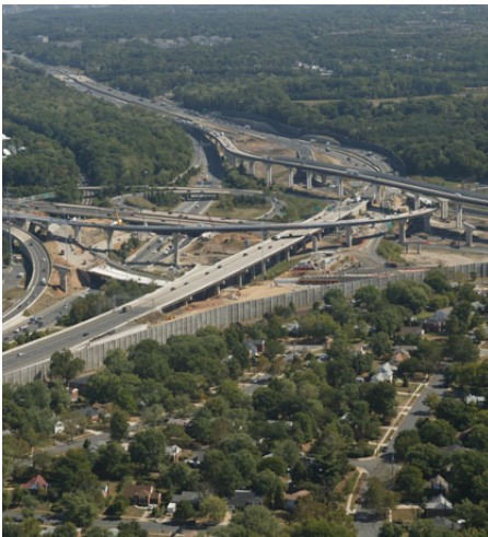
The Springfield Interchange Improvement Project met two critical milestones that will help ensure the entire project is completed in 2007 as scheduled.
