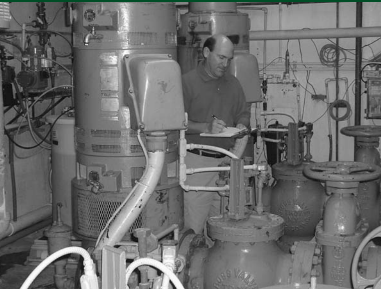
An ODW engineer inspects high service pumps at the Washington County Service Authority Water Treatment Plant as part of a semi-annual sanitary survey of the waterworks.
