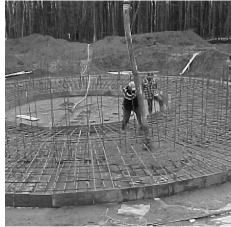
New Kent County borrowed 17,675,000 through the VPFP to finance improvements to the County's water and sewer systems, including the construction of water and sewer facilities to serve the Bottoms Bridge Service District area. New Kent County was able to save $87,281 per year by financing through the VPFP.
