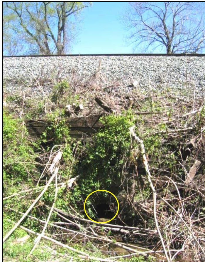
Photo 4-6: Drainage structure (obscured by vegetation) under track. Such structures will require extension or replacement as part of third track construction.
