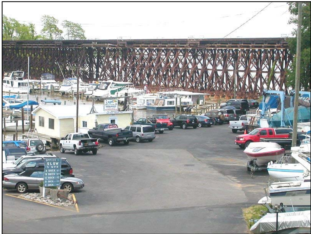
Photo 4-3: CSX Bridge at approximately MP 84.9 over Neabsco Creek which is considered a LARGE railroad bridge for purposes of this study.
