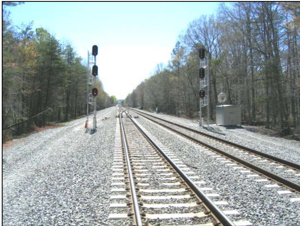
Photo 4-10: New concrete universal crossover and related signals at Arkendale Interlocking. Third track construction will require moving at least one signal column at both ends of the interlocking.
