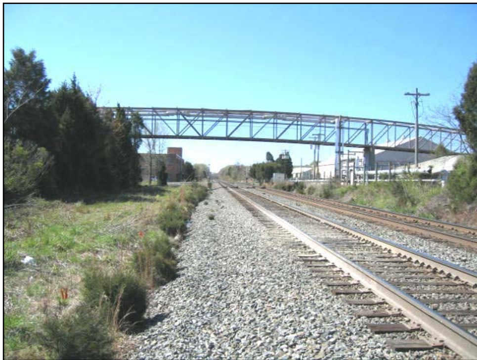
Photo 4-4: Pedestrian Bridge over CSX at approximately MP 76.8 which is considered without conflict for purposes of this study.
