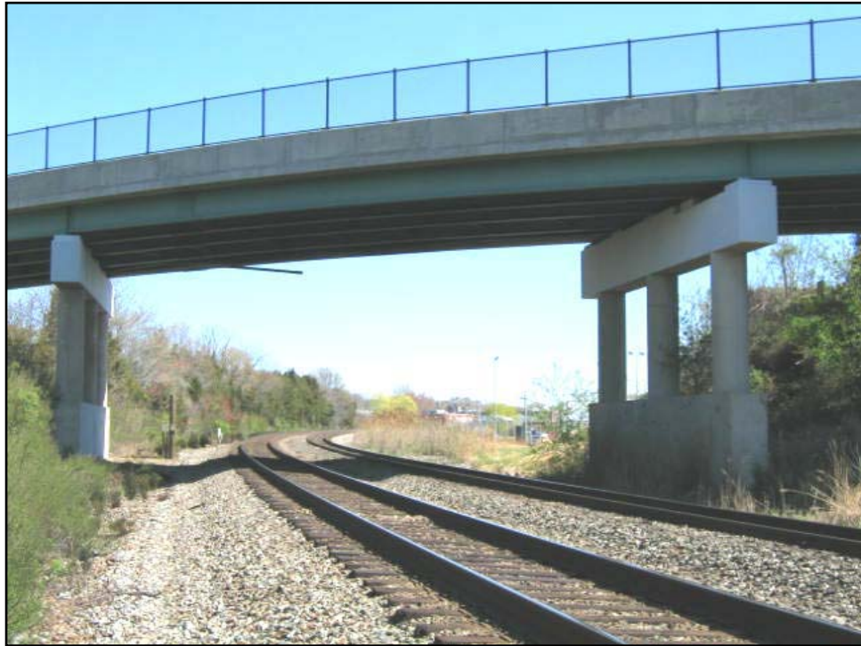
Photo 4-5: Range Rd. over CSX at approximately MP 77.5 which is considered a major conflict for purposes of this study. The skewed piers may be as little as 16-feet from existing centerline of track.
