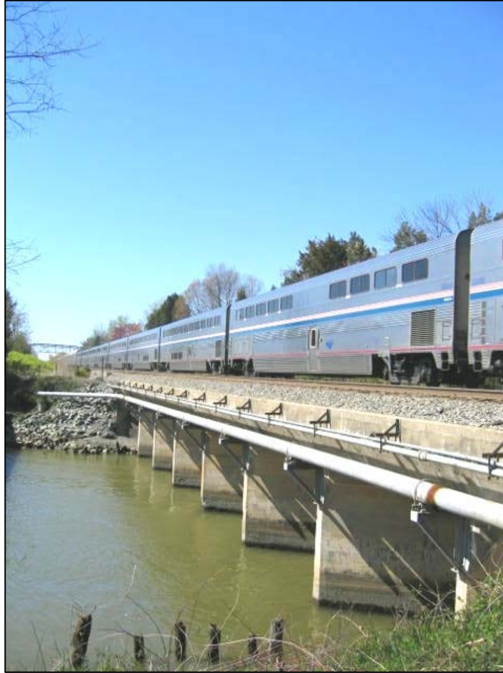
Photo 4-2: CSX Bridge at approximately MP 76.9 over Chopawamsic Creek which is considered a MEDIUM railroad bridge for purposes of this study.
