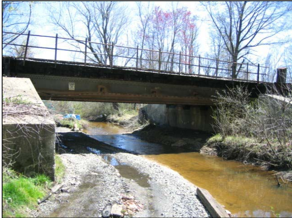
Photo 4-1: CSX Bridge at approximately MP 74.3 over a private road and un-named stream. This bridge is considered a SMALL railroad bridge for purposes of this study.
