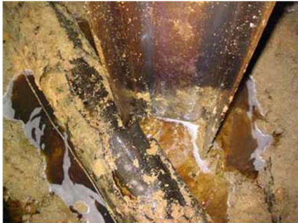
Fluid Leak After Pile Driver Struck Cable
