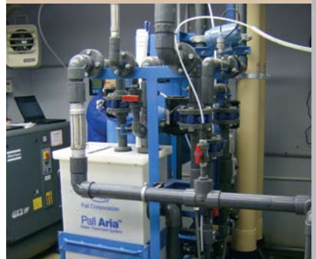
Augusta County SA new filtering system
