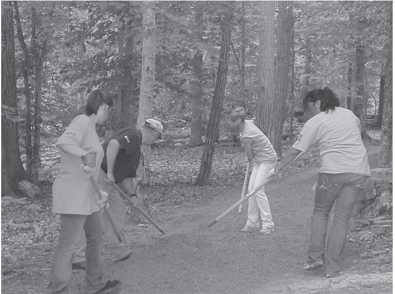
Youth Conservation Corp members and a crew supervisor working on Beaver Lake Trail at Pocahontas State Park during the summer education and community service program
