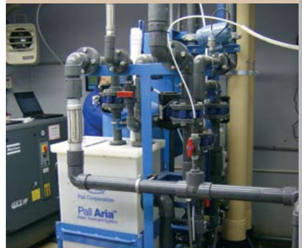
Augusta County SA new filtering system
