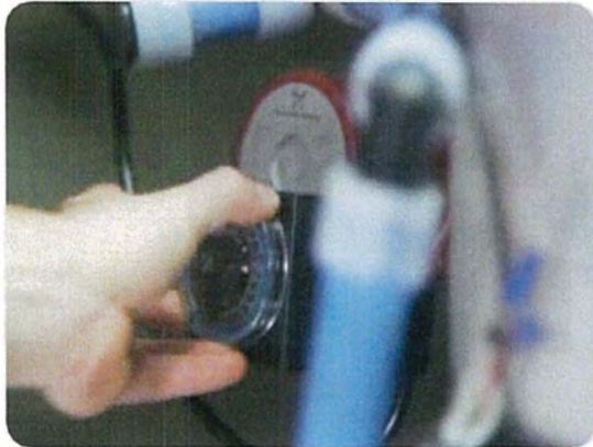
Video: adjusting the hot water heater V/O: after adjusting the water temperature
