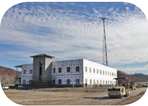
The Crooked Road Technology Center, a 45,000 sq. ft. multi-tenant facility, takes shape in the Scott County Regional Business and Technology Park in Duffield.
