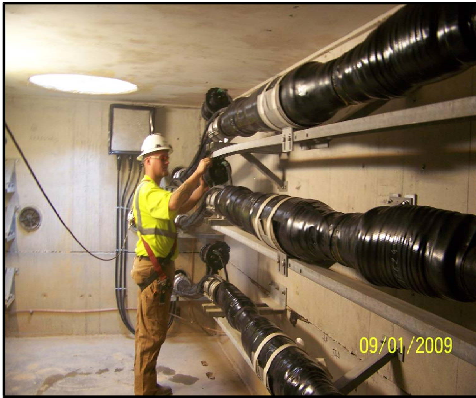
Figure 17: View of vault interior and cable splice along Garrisonville underground transmission line.
