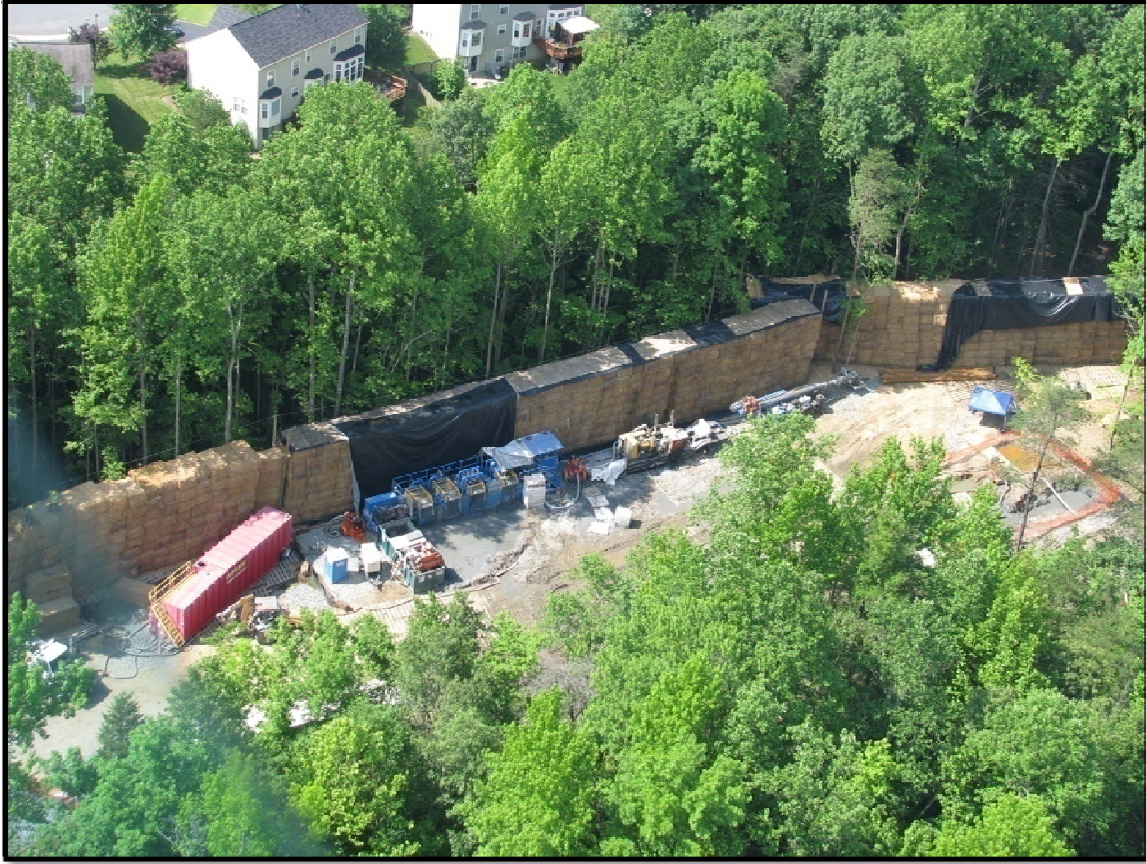
Figure 10: View of sound-insulating wall proximate to drilling site near Garrisonville underground line.
