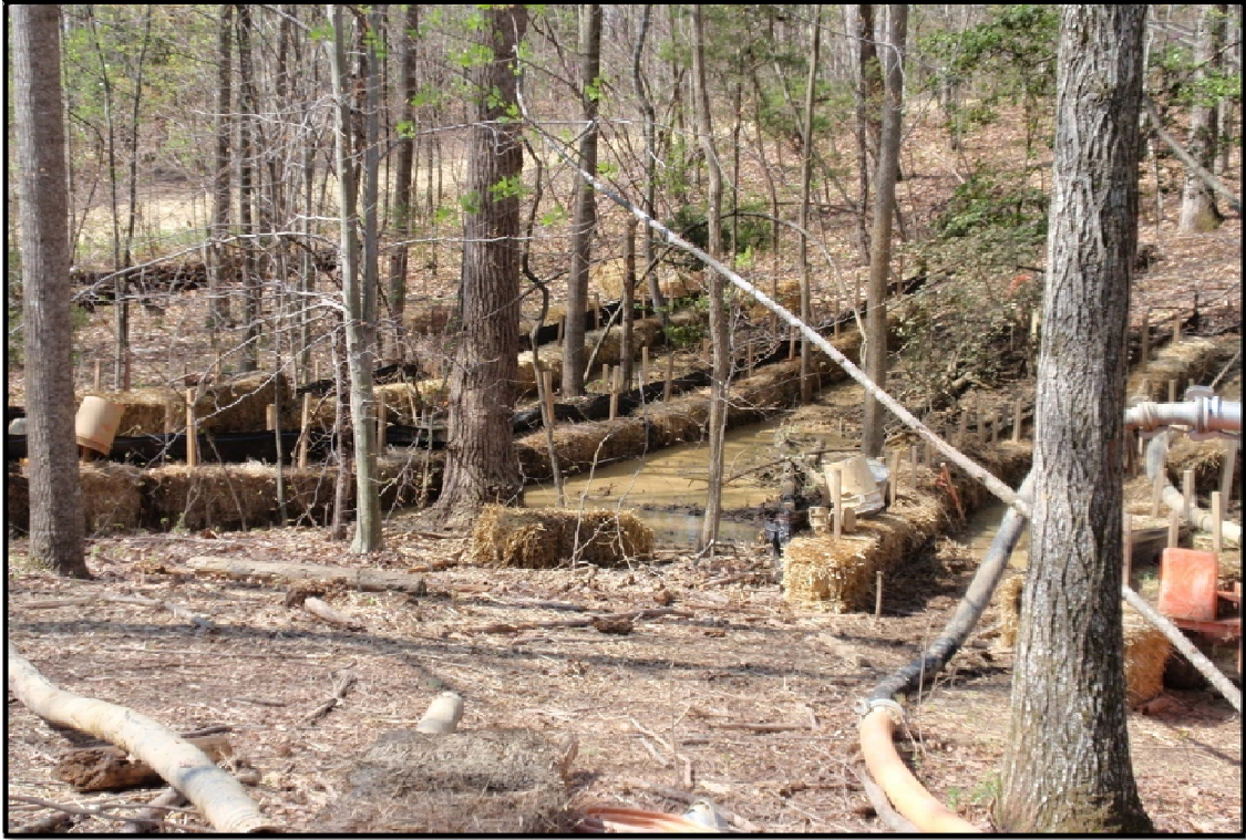
Figure 9: Site of frac-out showing containment measures for the protection of the environment.
