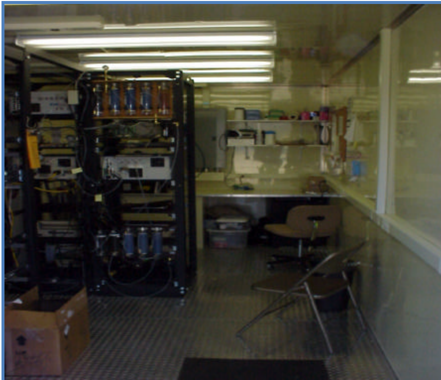
Figure 2-3: Interior View of the Henrico County NATTS/NCORE Site
