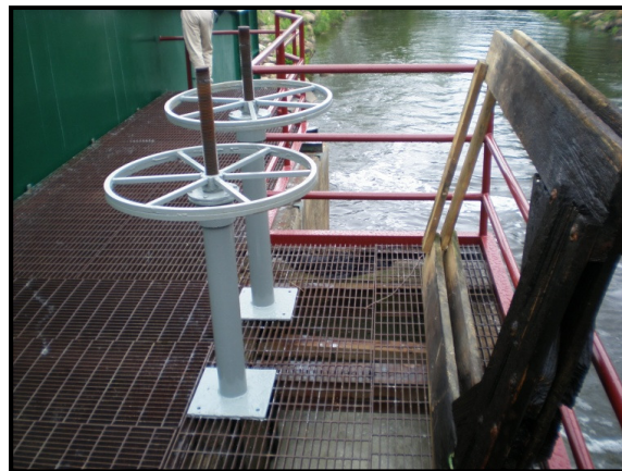
Figure 5 Photo of Gate Valves to Attraction Flow Chambers
