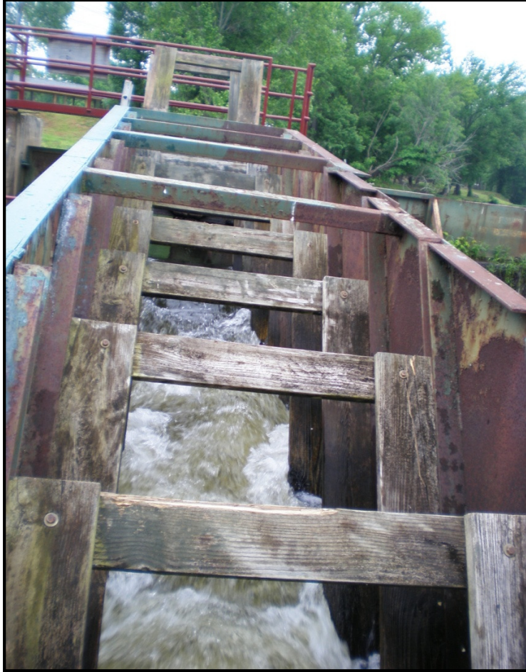
Photo 7 Standing near turning pool of Denil fishway looking upstream at baffled chute
