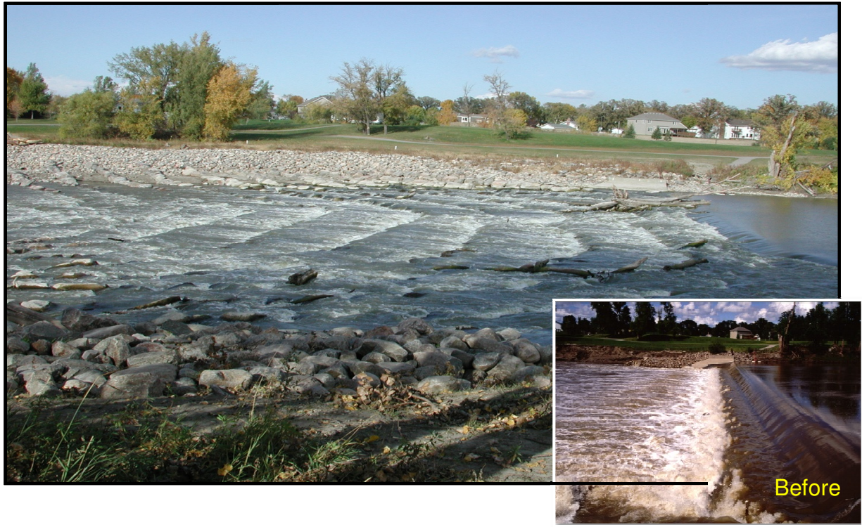
Figure 17 Before and after Photos of Rock Ramp Fishway Constructed at Riverside Dam (Photos courtesy of Dr. Luther Aadland).
