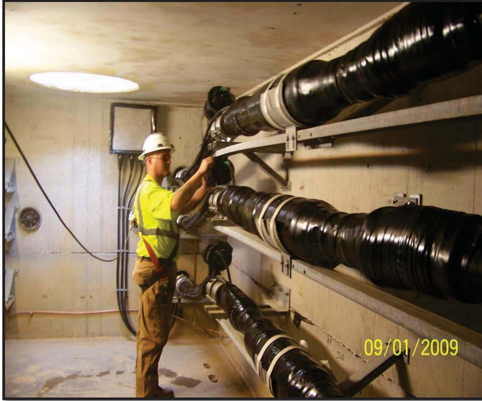
Figure 17: View of vault interior and cable splice along Garrisonville underground transmission line.
