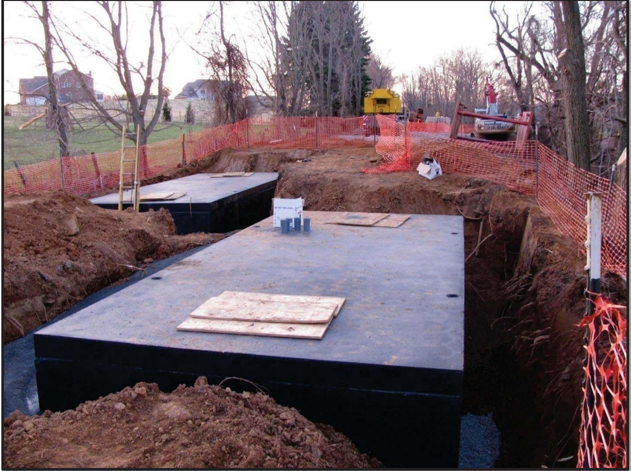
Figure 2: Manholes "6A" and "6B." Once restored, the W&OD Trail will thread between the four manhole lids on the surface.
