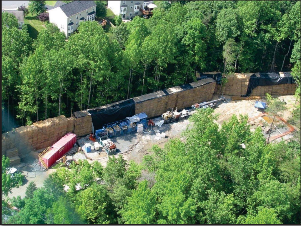
Figure 10: View of sound-insulating wall proximate to drilling site near Garrisonville underground line.
