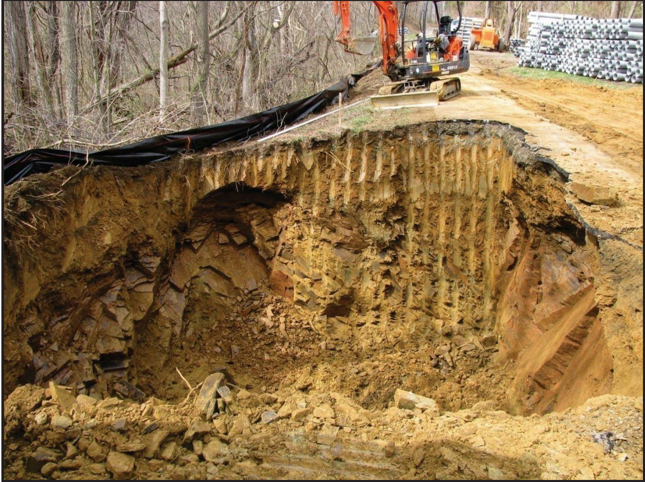
Figure 4: Layers of dense rock below and beside the original trail (top right). Stacks of conduit (pipe) also visible.
