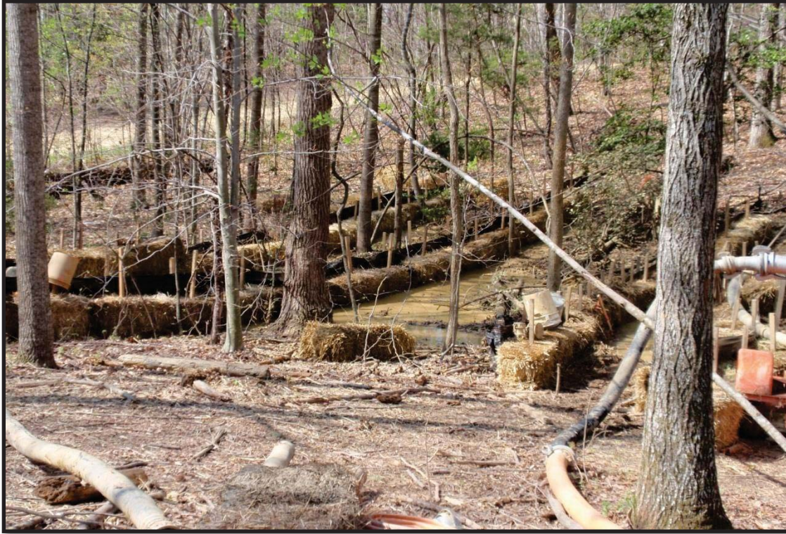
Figure 9: Site of frac-out showing containment measures for the protection of the environment.
