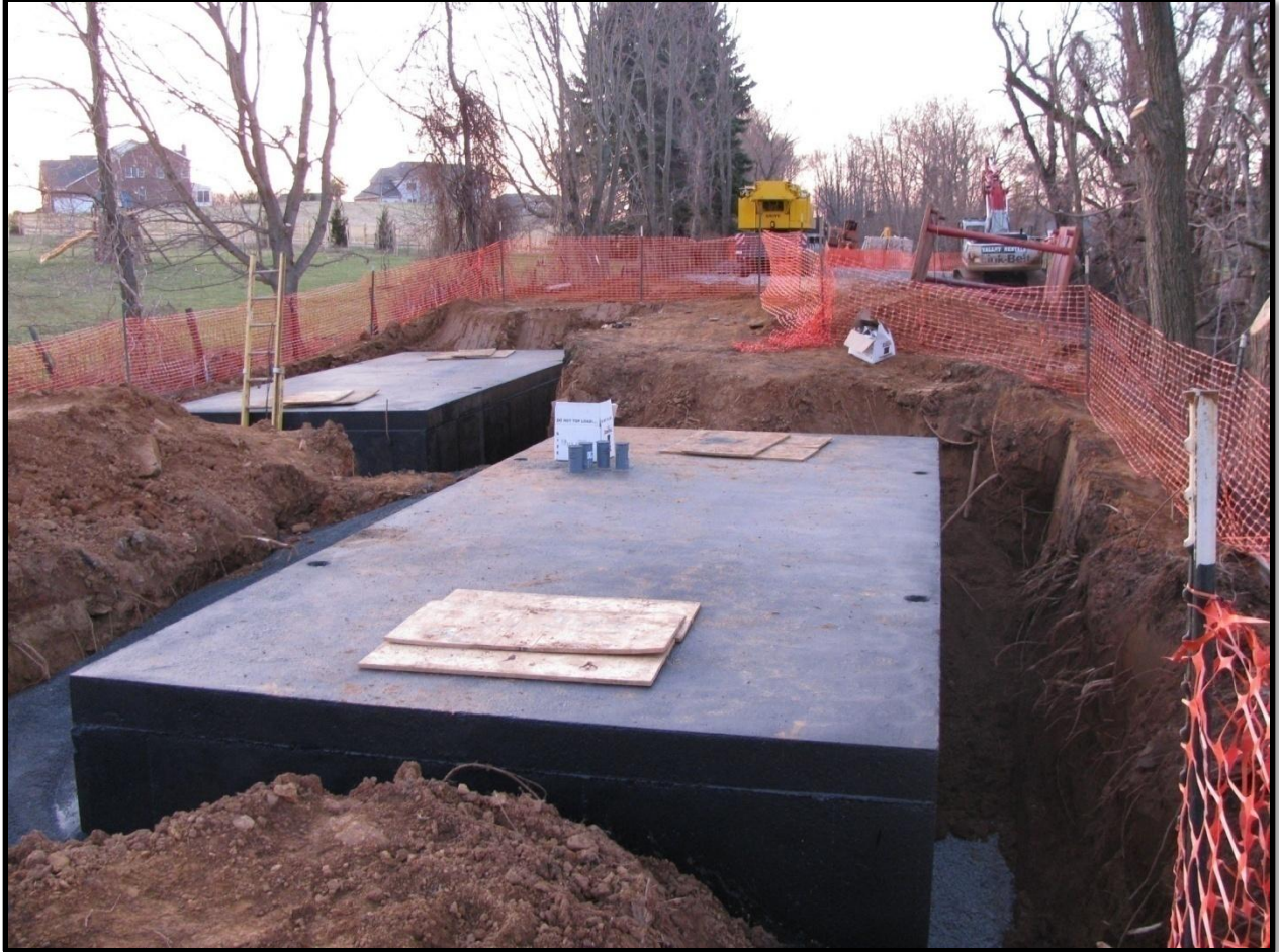
Figure 4: Manholes "6A" and "6B." Once restored, the W&OD Trail will thread between the four manhole lids on the surface.
