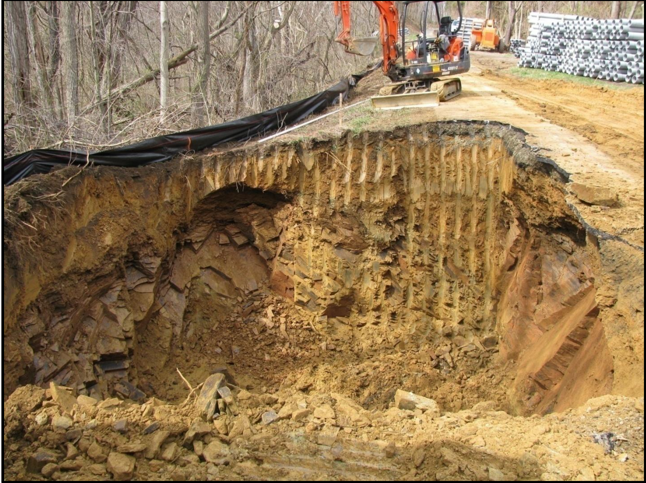
Figure 6: Layers of dense rock below and beside the original trail (top right). Stacks of conduit (pipe) also visible.
