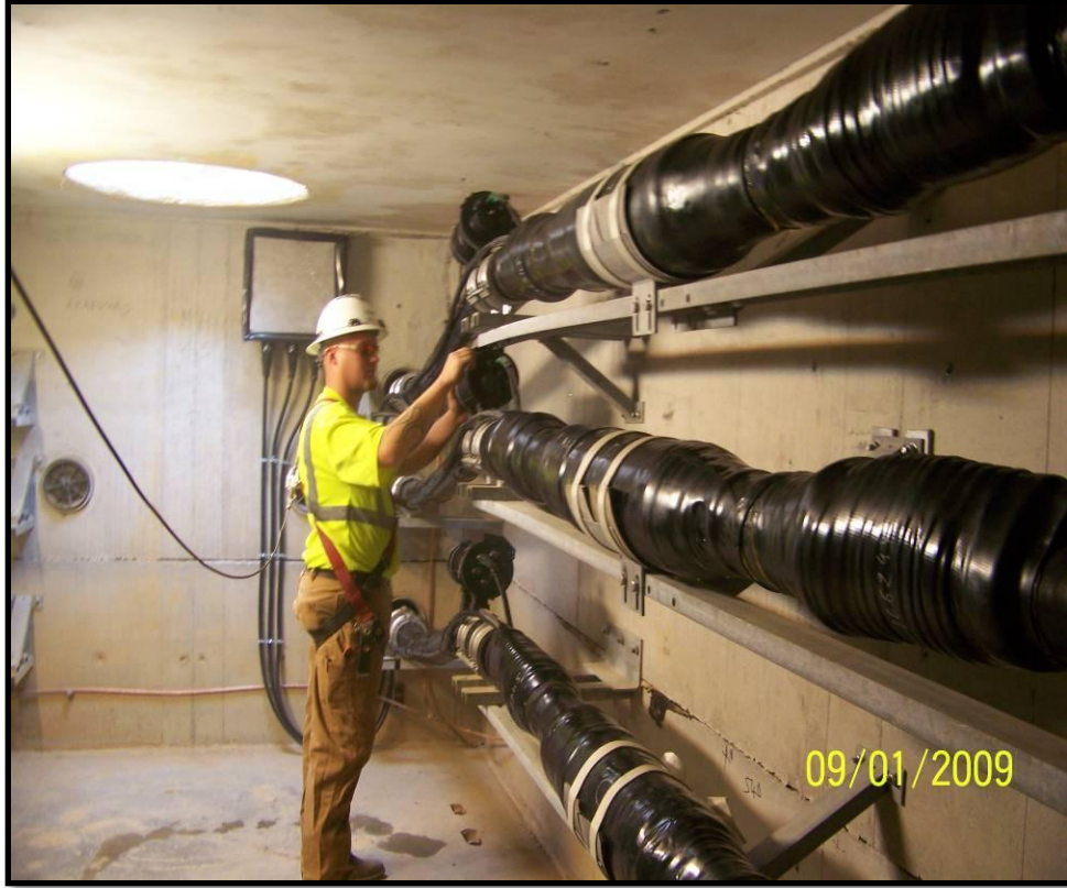
Figure 19: View of vault interior and cable splice along Garrisonville underground transmission line.
