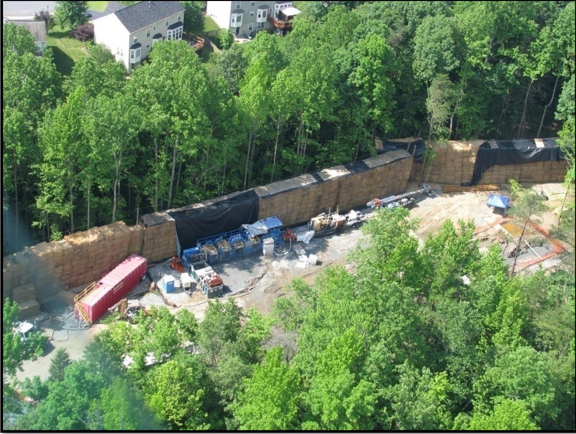
Figure 12: View of sound-insulating wall proximate to drilling site near Garrisonville underground line.
