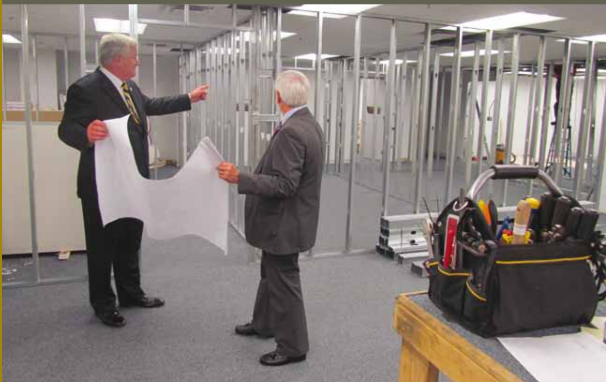
Director and Chief Randall L. Clouse, Deputy Director of Investigations and Audit Paul Anderson Construction underway to make room for expanding MFCU.
