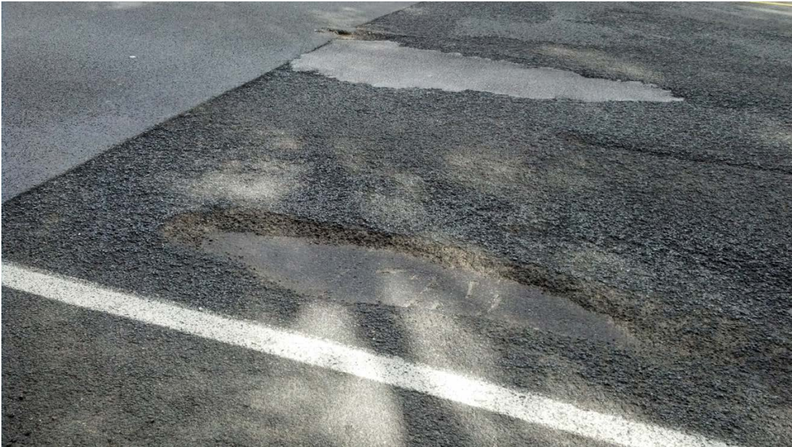
Figure 9. PFC Failure Due to "Cold Start"- Route 7.
