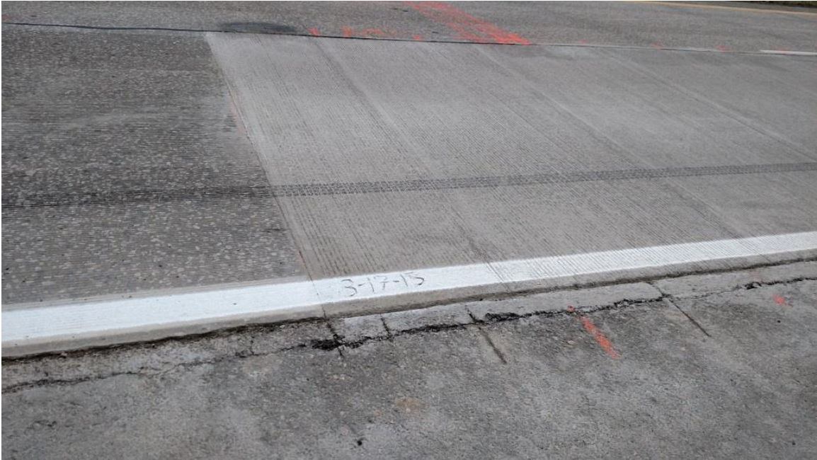
Figure 11. New Concrete Repair in Quiet Concrete Project - Route 76. The darker material to the left is NGCS. The patch to the right has been transversely tined. Note date on new patch (3-17-2015).
