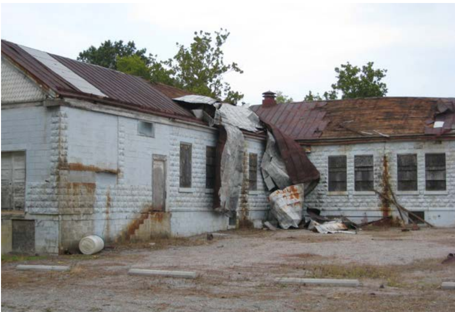
The Work Activities Building No. 11 at Central State Hospital. Budget constraints on many agencies leave little funding for routine maintenance or stabilization of vacant buildings. (Photo: DHR)
