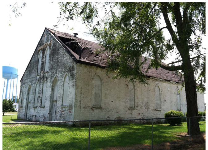
The Chapel at Central State Hospital before the roof caved in.
