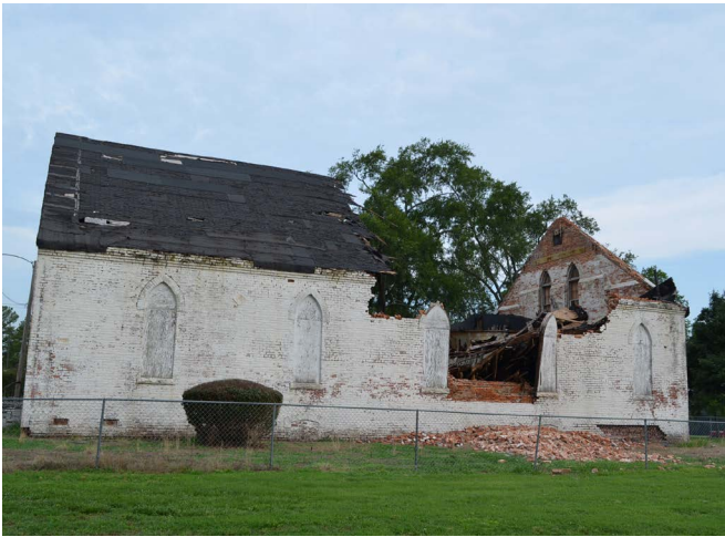
The Chapel at Central State after the roof collapsed in 2014. (Photos: DHR)
