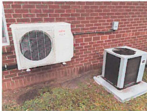
Photo of new mini-split heat pump (left) and the existing heat pump (right)
