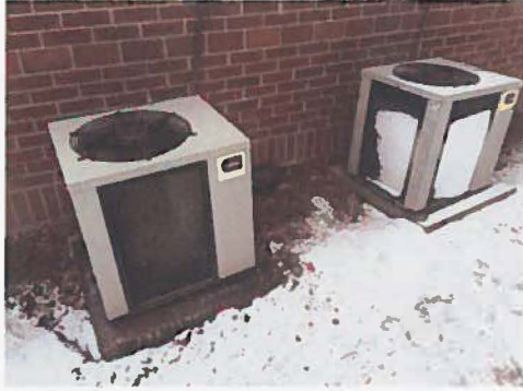
Ice build-up on the existing HVAC units indicated the units were not operating efficiently
