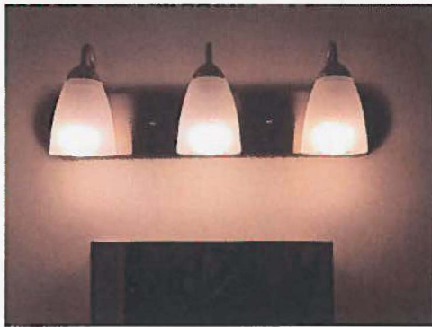
New LED lighting
