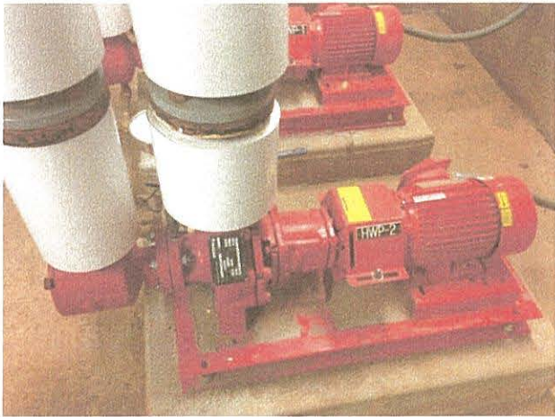
Hot Water Pumps - Typical
