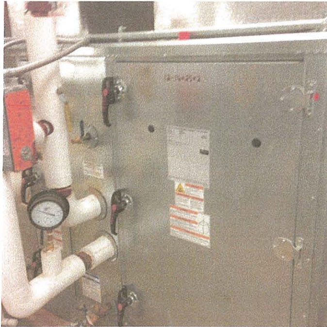
Attic Air Handling Unit-Typical
