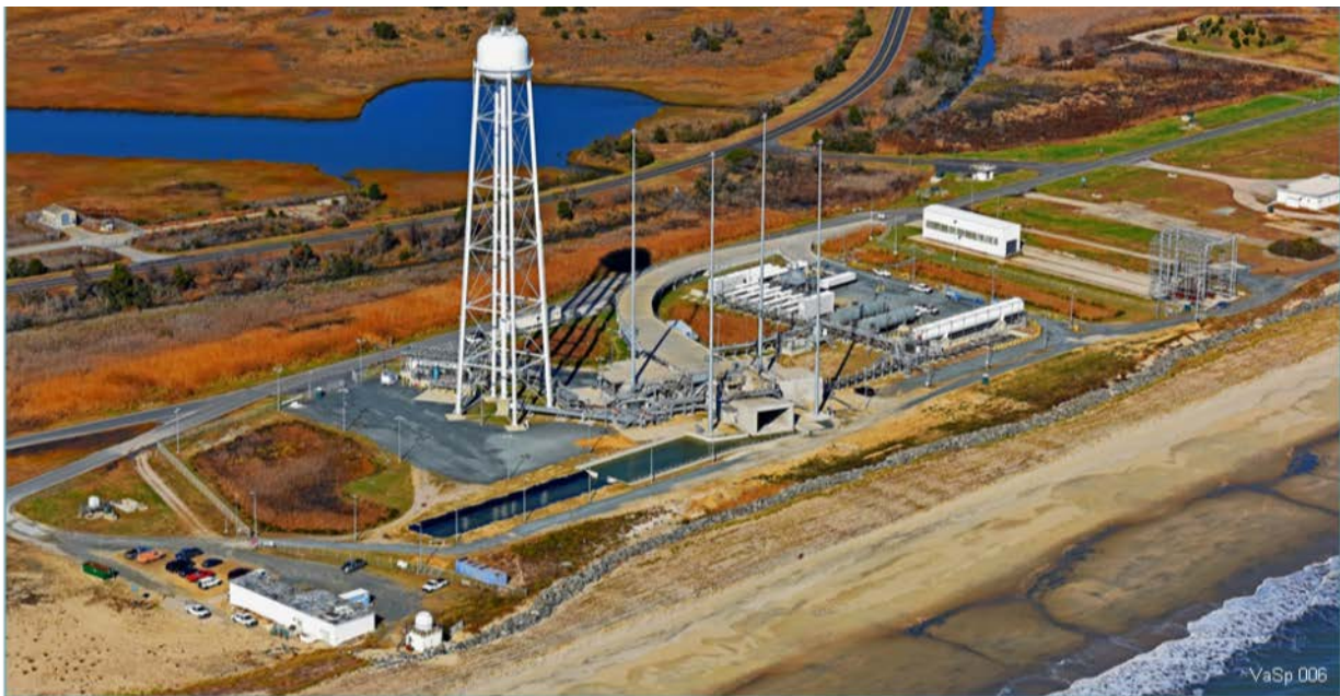
Figure 2-3. Launch Pad Repair. Repair of Pad 0A was completed ahead of schedule to support future flight efforts.
