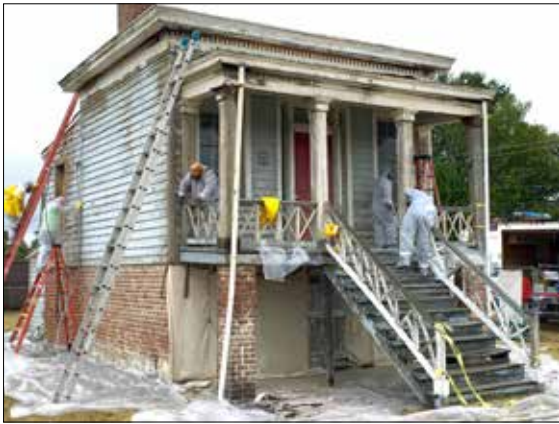
After removing modern siding, volunteers work to strip away old lead paint.
