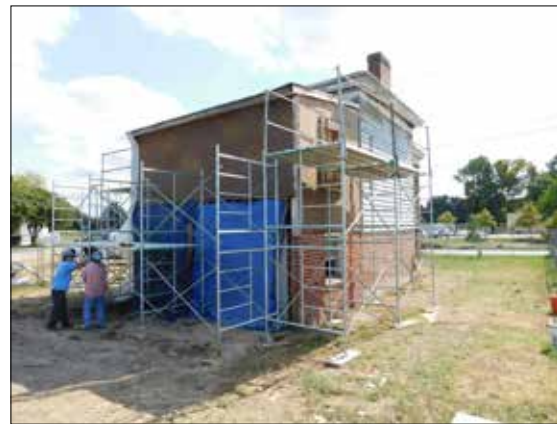
After removal of the rear addition, scaffolding was set in place to allow repointing and repair of siding.
