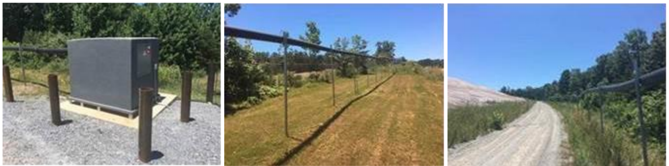
Figure 3. – Vapor-Phase Odor Neutralization System
