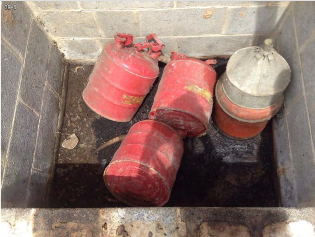
Photo 27-2 Gasoline and oil containers within concrete block structure outside Building 39, heavy petroleum staining on bare dirt floor.
