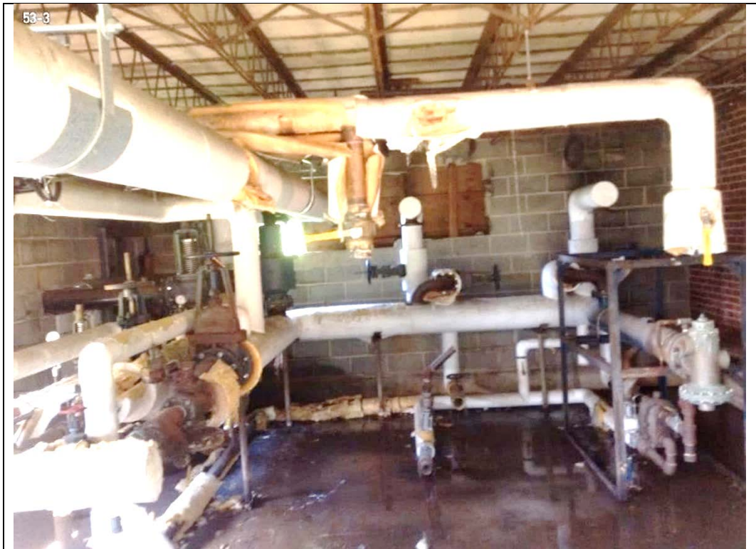
Photo 28-3 Terminated and modified piping with Building 53 indicates a prior boiler or arrangement.
