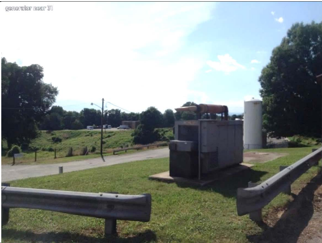
Photo 33-1 1,000-gallon diesel UST and backup power generator at Building 31
