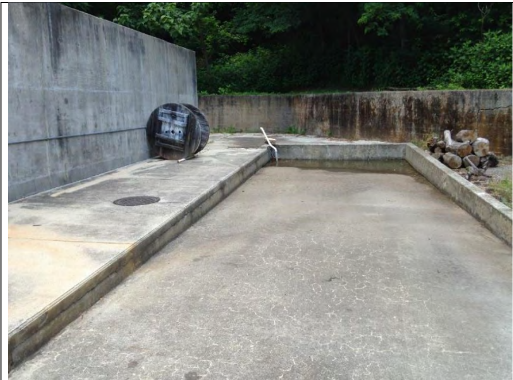
Photo 3-3 Offloading area for tanker trucks, 90,000-gallon No. 2 Heating Oil AST at the boiler plant, Building 77
