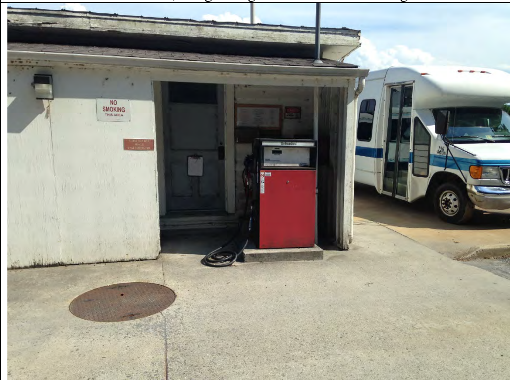
Photo 30-2 Dispenser above 8,000-gallon gasoline UST at Building 36
