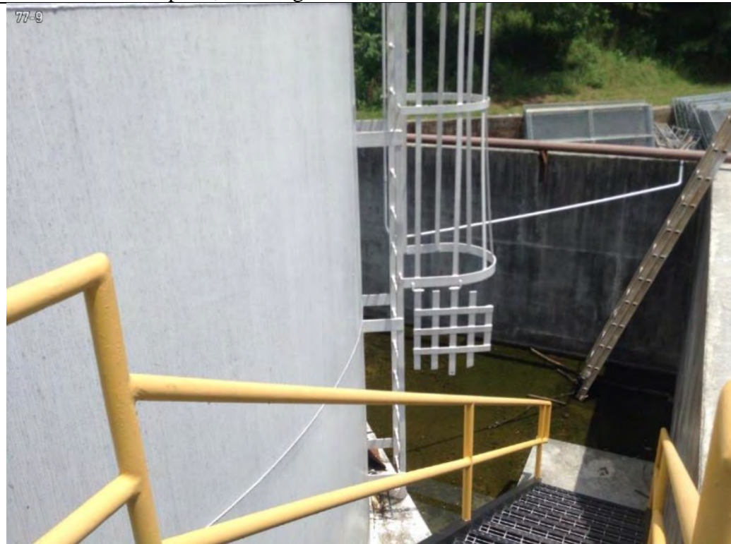
Photo 3-4 Standing water within containment dike, no petroleum sheen evident
