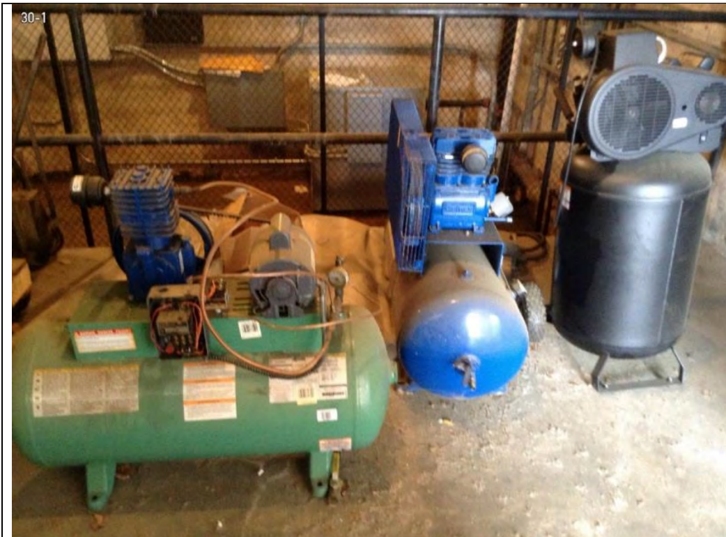
Photo 38-1 Air compressor storage in lower level of Building 30
