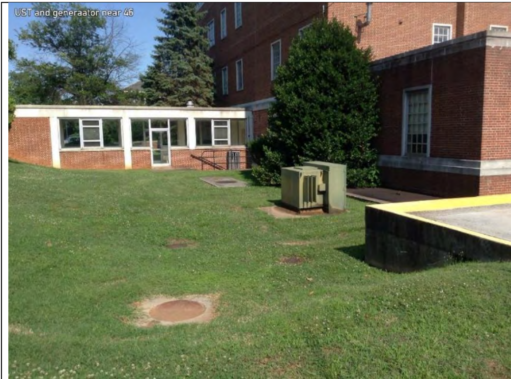
Photo 29-1 1,000-gallon diesel UST for generator within basement of Building 46
