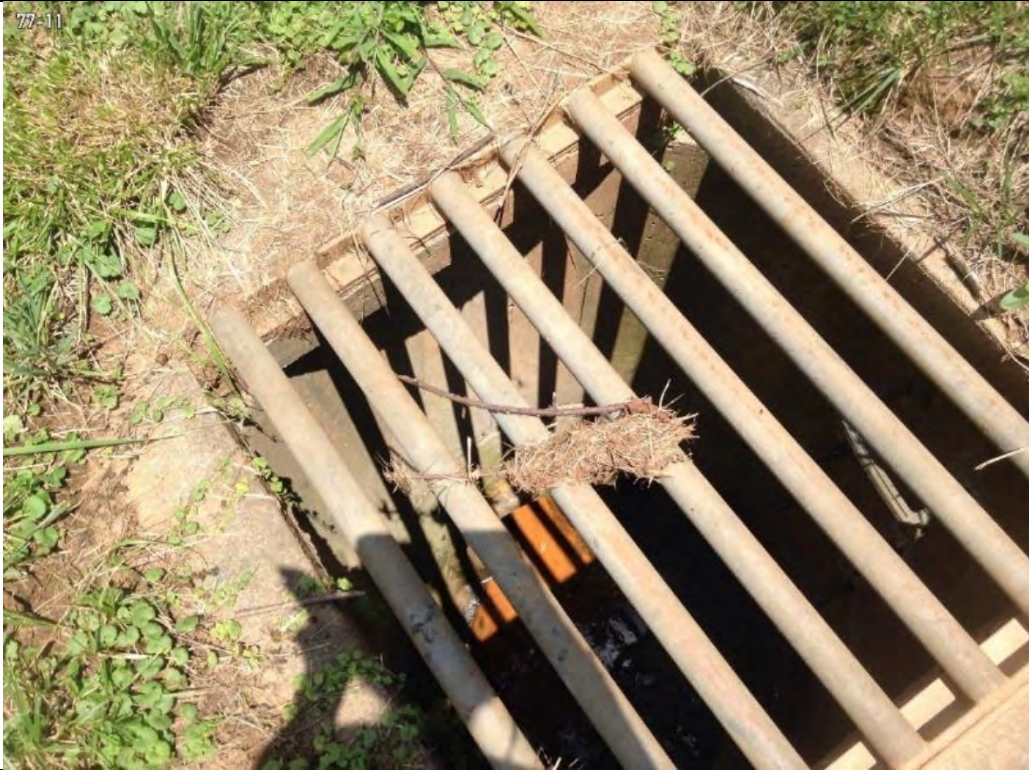
Photo 9-2 Storm water drop inlet at boiler plant (Building 77), no current visual evidence of fines or other coal related impacts.
