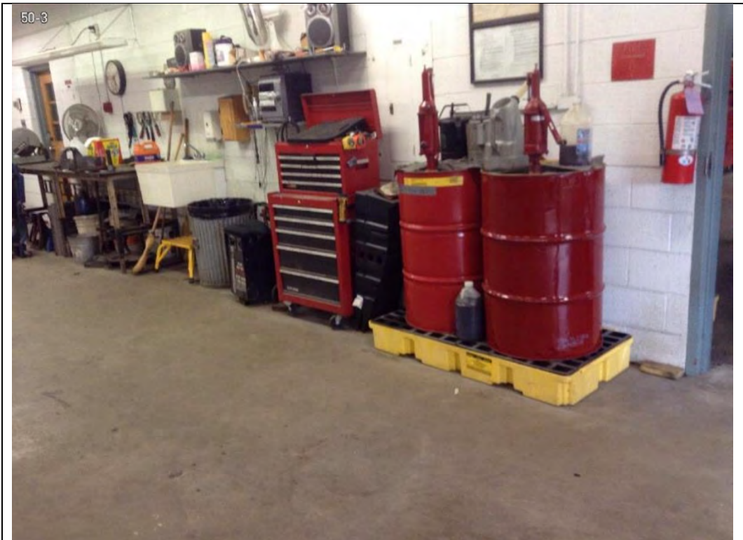
Photo 37-1 New motor oil drums on spill pallets within vehicle maintenance bays in Building 50
