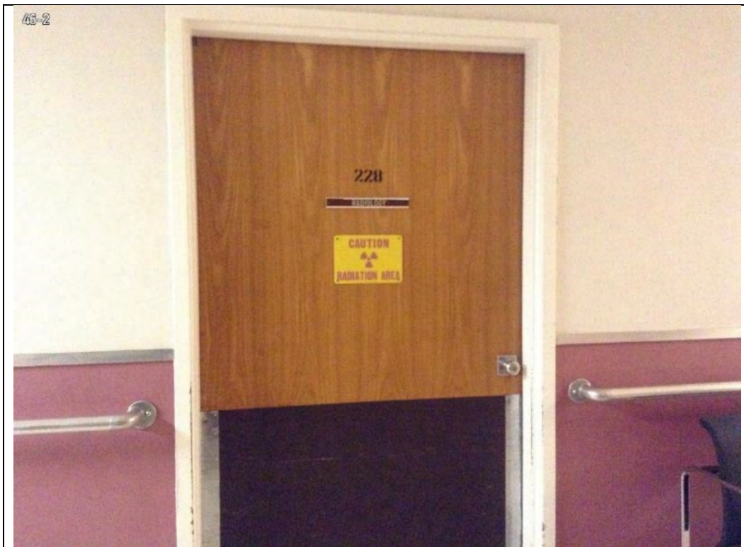
Photo 5-3 Entrance to X-ray in Building 46. All appurtenances in use, clean, and well maintained.
