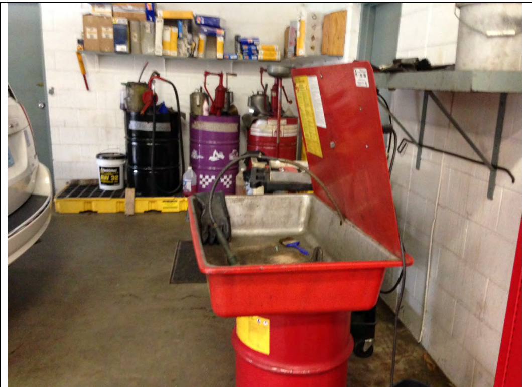
Photo 37-3 Parts washer and new motor oil drums on spill pallets within vehicle maintenance bays in Building 50
