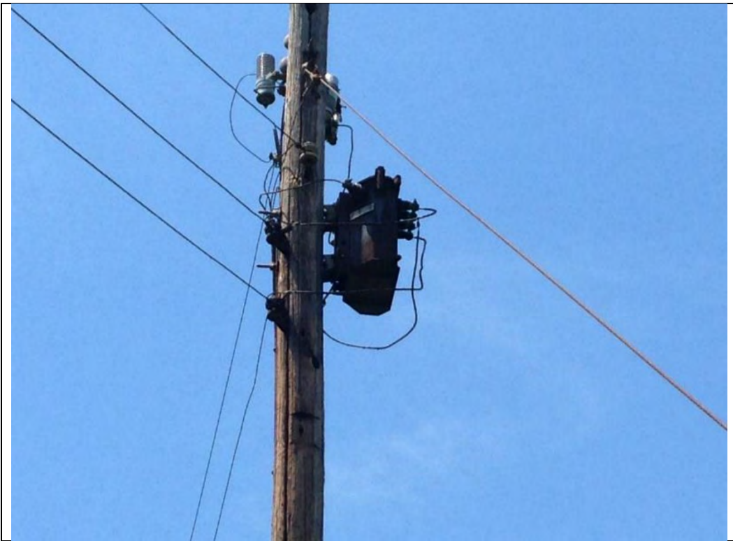
Photo 11-6 Pole-mounted transformer outside incinerator Building 13, not in use and suspect PCB-containing due to age and design.
