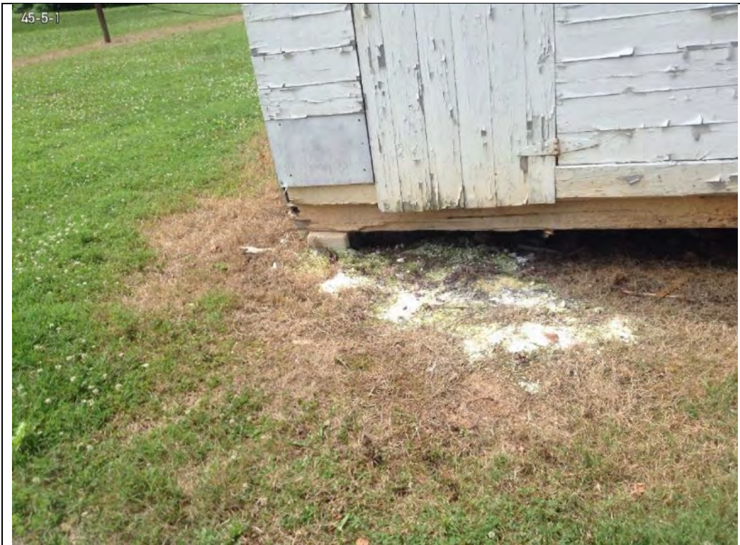
Photo 36-1 Spilled chemical and associated dead vegetation outside storage Building 45-5
