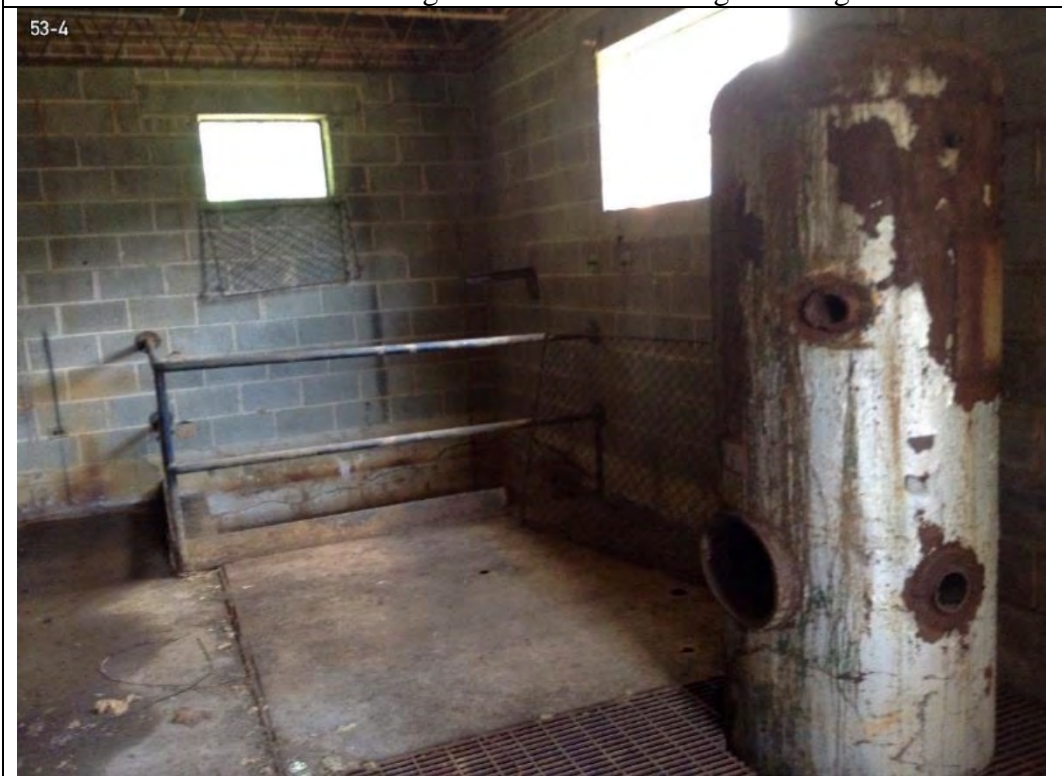
Photo 28-2 Former boiler tank (no longer used for existing system) in Building 53
