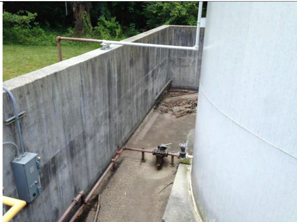
Photo 3-2 Interior of containment dike, 90,000-gallon No. 2 Heating Oil AST at the boiler plant, Building 77
