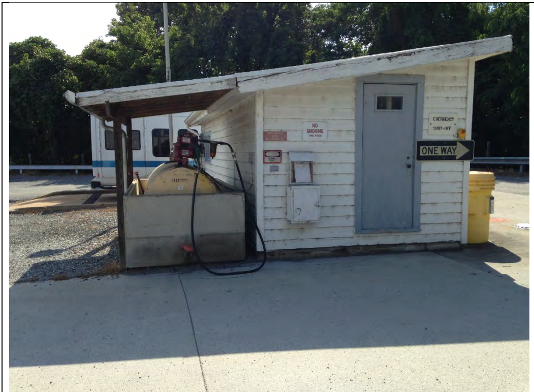
Photo 1-1 View of Diesel AST at Building 36, looking west. No evidence of staining or odors around tank.
