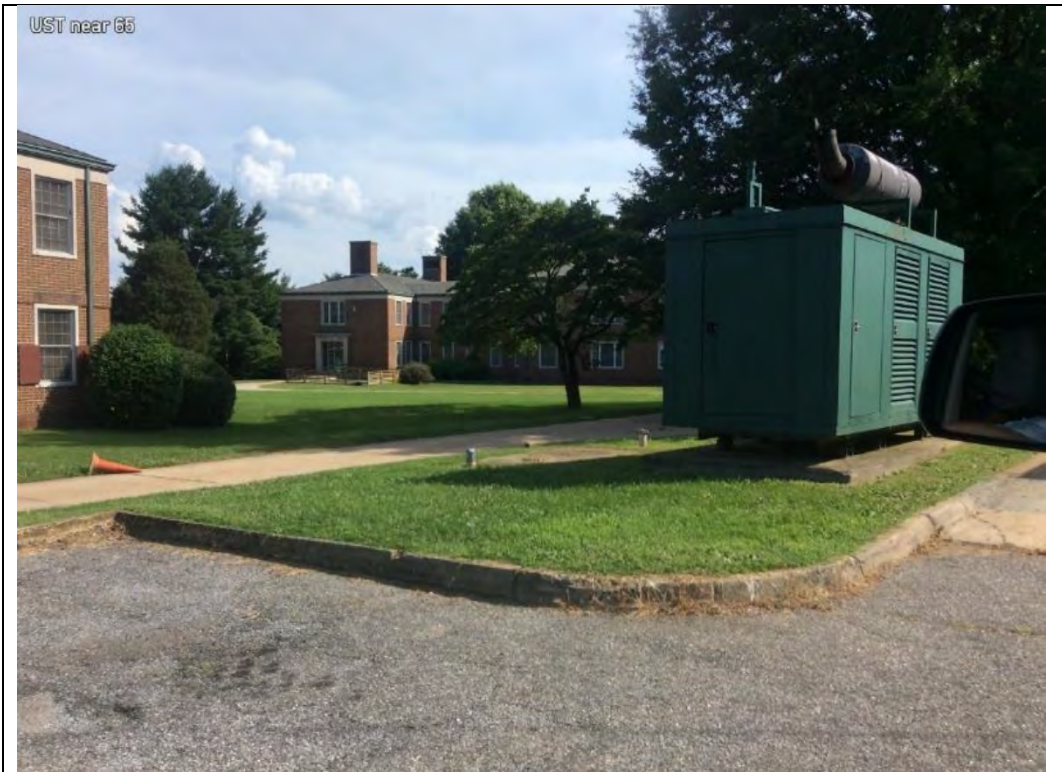
Photo 31-1 1,000-gallon diesel UST and backup power generator at Building 65
