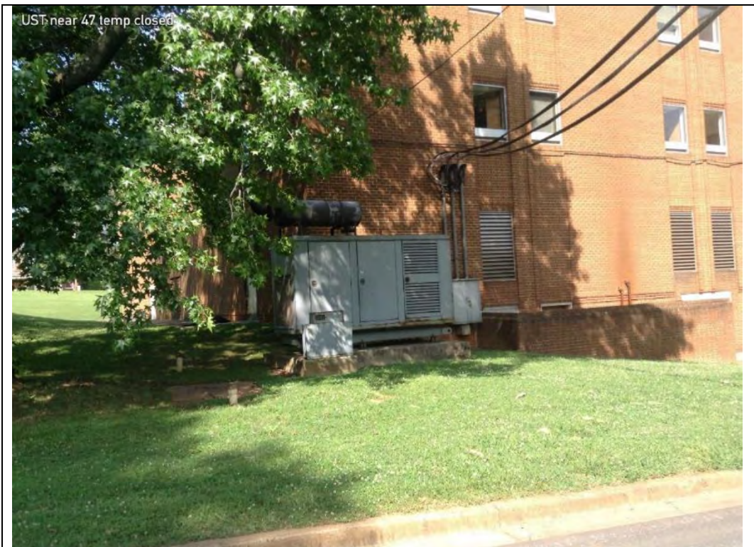
Photo 32-1 1,000-gallon diesel UST and backup power generator at Building 47
