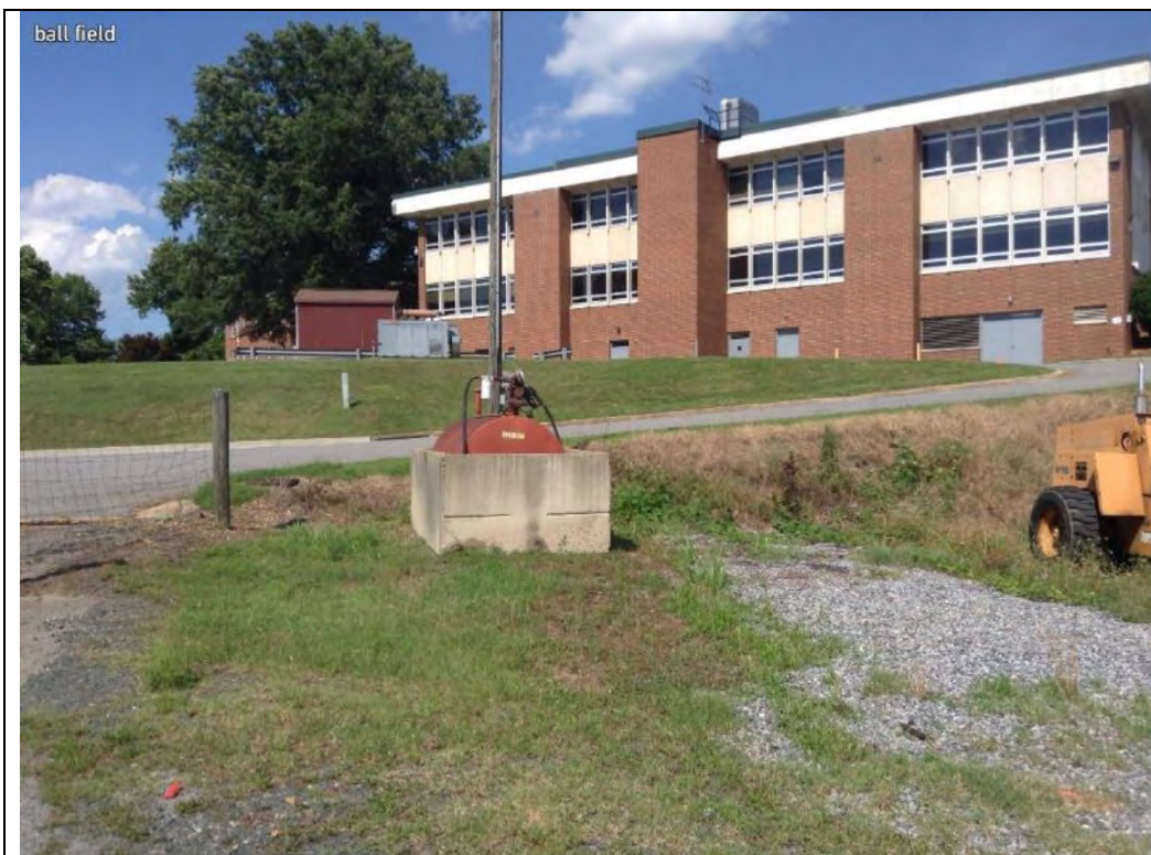
Photo 2-1 View of Diesel AST at equipment yard commonly referred to as the former “ball field,” looking east towards Building 31. No evidence of staining or odors around tank. This AST was formerly located at the grounds crew Building 37.
