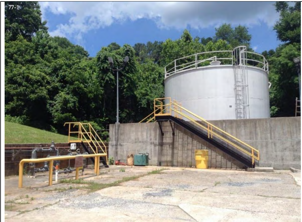
Photo 3-5 Additional view of 90,000-gallon No. 2 Heating Oil AST at the boiler plant, Building 77
