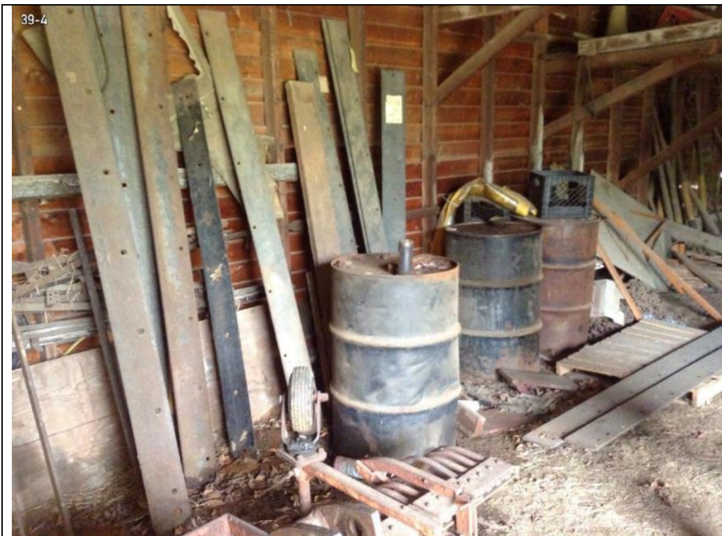
Photo 27-1 Drums of used motor oil with visual indication of spills onto the surrounding dirt floor within Building 39
