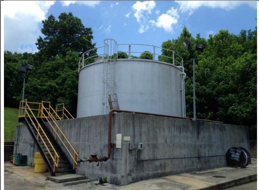
Photo 3-1 View of 90,000-gallon No. 2 Heating Oil AST at the boiler plant, Building 77.
