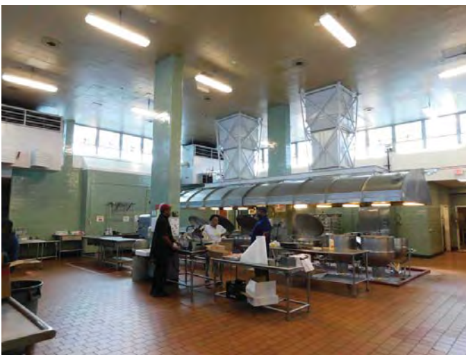
R16: HEATING & VENTILATING UNITS, NO LONGER OPERABLE, LEAK WATER, Photo 633
