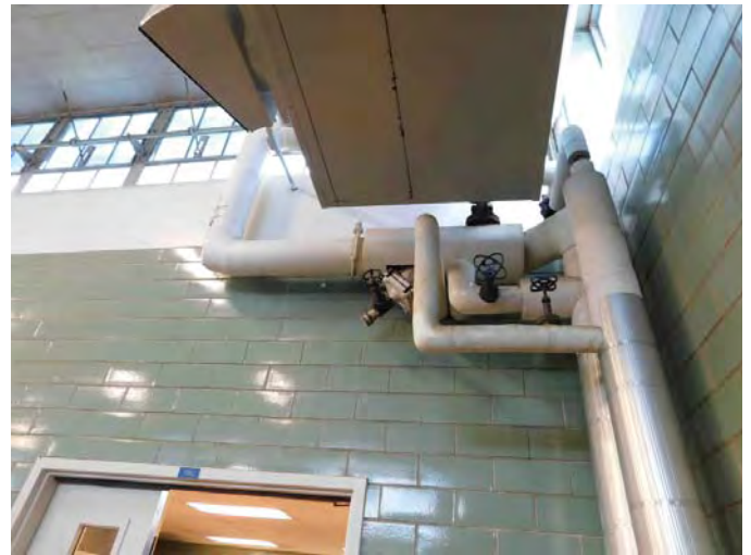
R16: KITCHEN HEATING & VENTILATING UNIT, NO LONGER OPERABLE, LEAKS WATER, Photo 751
