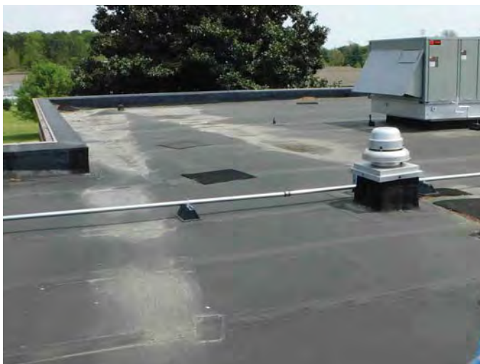
R3: LOW SLOPE MEMBRANE SYSTEMS, VIEW TO EAST, EVIDENCE OF PONDING WATER, Photo 784
