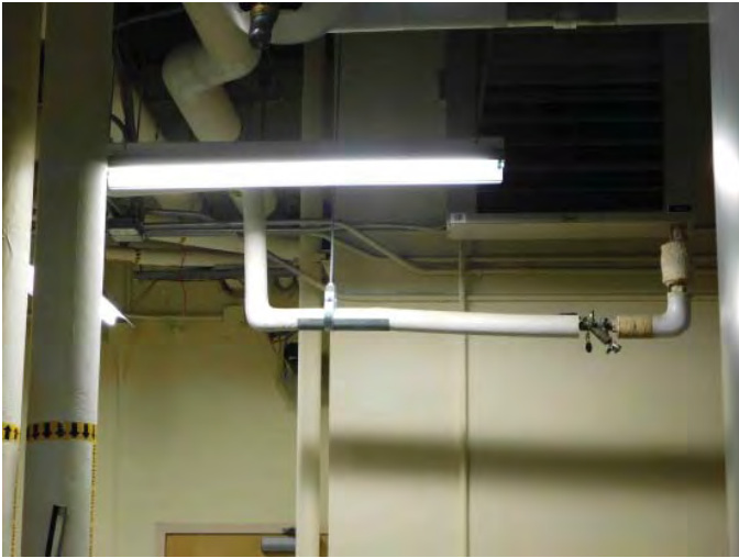
R4: SAGGING CVPC PIPING
