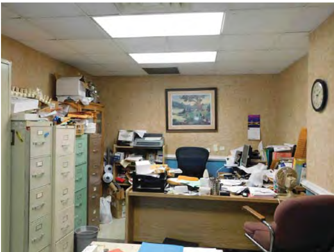
R5: CEILING FINISHES, CEILING TILE REPLACEMENT & ITEMS ABOVE FLOOR, DUE TO WATER INFILTRATION, RM 103, BUCKET ON FLOOR TO CATCH WATER, Photo 836
