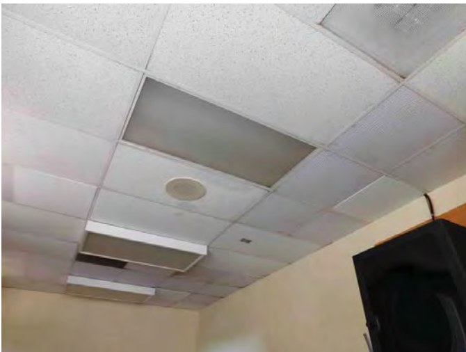
R5: CEILING FINISHES, CEILING TILE REPLACEMENT DUE TO WATER INFILTRATION, RM 103A, LEAK ABV AUDIO VISUAL EQUIPMENT, Photo 1158
