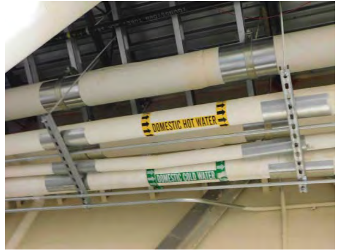
R4 SAGGING CVPC PIPING
