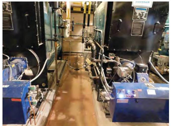
R6a: BOILER DRAIN FOR FLUSHING, SEDIMENT ON FLOOR DUE TO FLOODING
