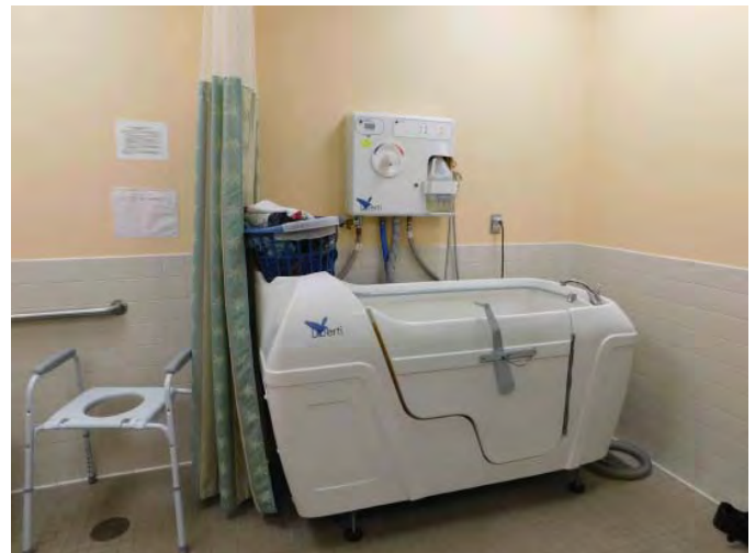
R2: LIBERTI TUB. ALL BATHTUBS LEAK THROUGH THE DOOR CLOSURE SEAL. Photo 1489
