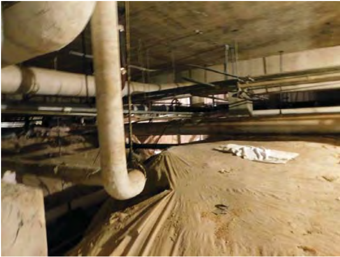
R10 & R10A: DOMESTIC PLUMBING IN CRAWL SPACE, Photo 851
