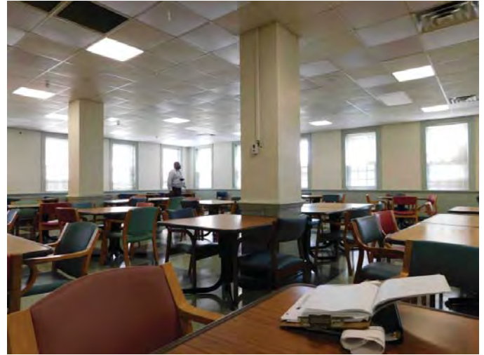
R5: CEILING FINISHES, CEILING TILE REPLACEMENT DUE TO WATER INFILTRATION, RM 102, Photo 731
