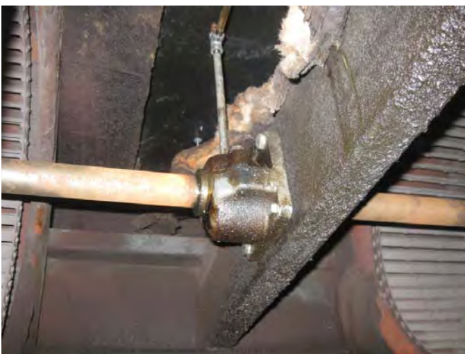
R12: BASEMENT H&V UNIT, H-3, COILS DAMAGED, BEYOND USEFUL LIFE,
