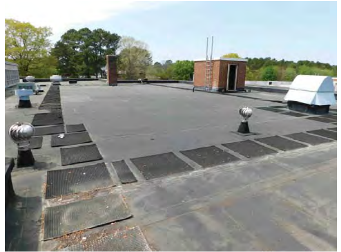
R3: LOW SLOPE MEMBRANE SYSTEMS, VIEW TO NORTH, EVIDENCE OF PONDING WATER, Photo 780
