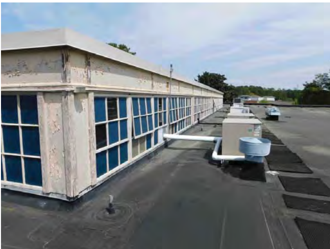
R2: REPLACE STEEL WINDOWS, SOME NO LONGER CLOSE, Photo 804
