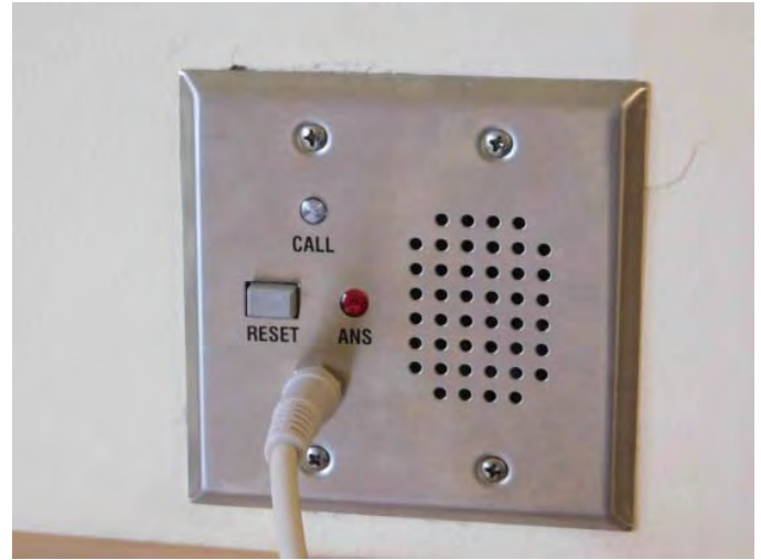
R8: NURSE CALL STATION, INOPERABLE & NEEDS TO BE REPLACED WITH ANTI-LIGATURE, Photo 1466
