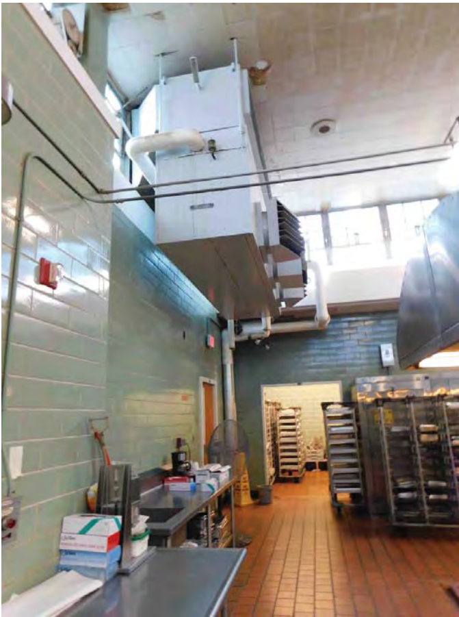
R16: HEATING & VENTILATING UNIT, NO LONGER OPERABLE, LEAKS WATER, Photo 637
