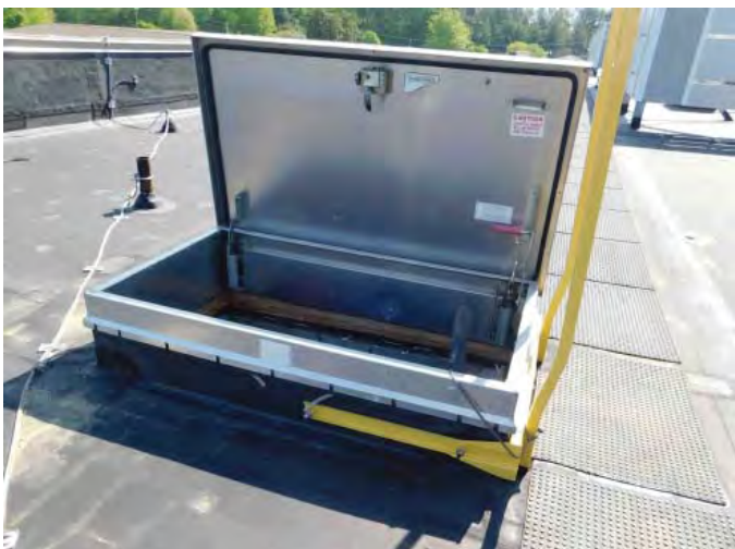
R1: TOP OF SHIP'S LADDER. LACK OF HANDRAIL AT TOP, Photo 1578d
