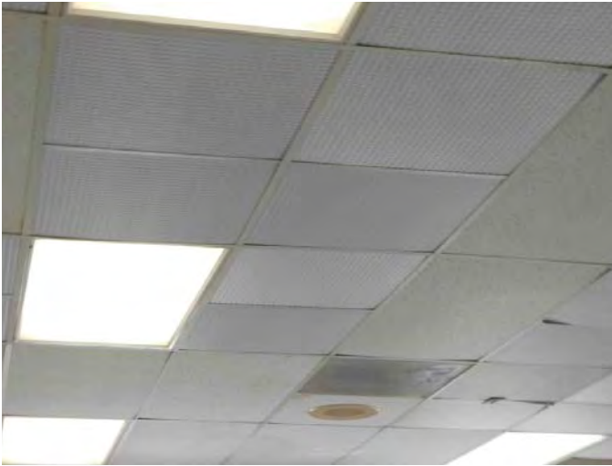
R5: CEILING FINISHES, RM 101A, REPLACEMENT CEILING TILES DUE TO WATER INFILTRATION, Photo 822
