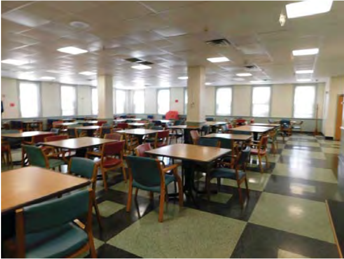
R5: CEILING FINISHES, CEILING TILE REPLACEMENT DUE TO WATER INFILTRATION, RM 102, Photo 724
