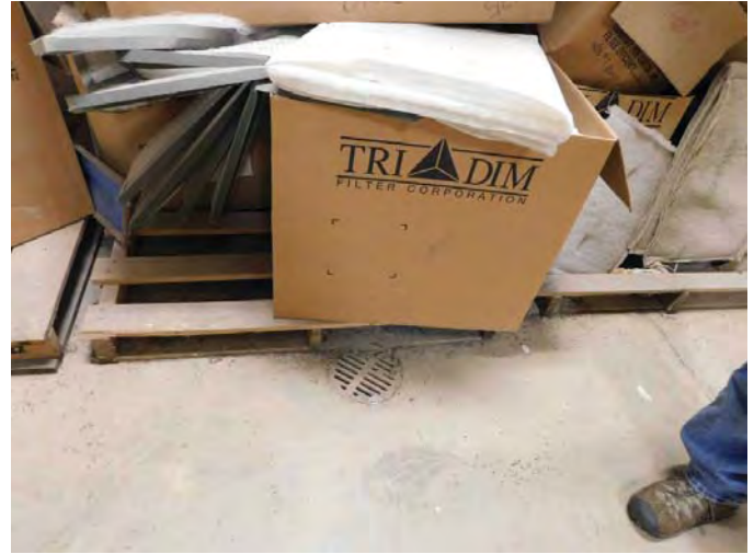
R6a: BOILER DRAIN FOR FLUSHING, N-S CORRIDOR, DRAIN, ELEVATED BOXES & SEDIMENT ON FLOOR DUE TO FLOODING
