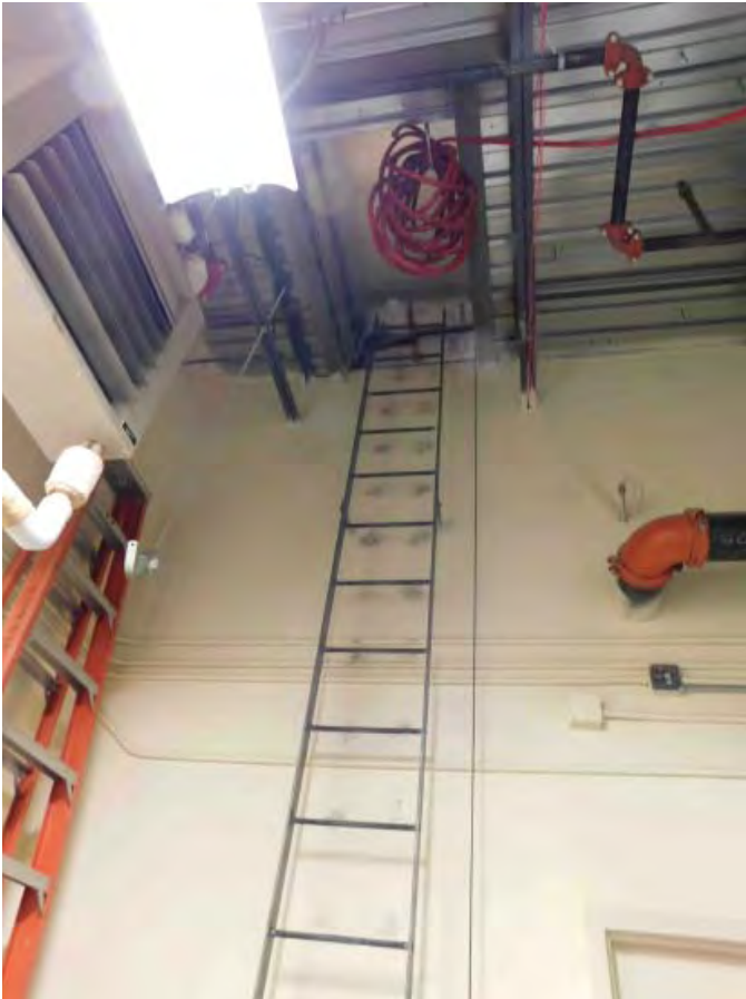
R1: SHIP'S LADDER, NO FLAT TREADS, HANDRAILS OR SAFETY CAGE, DIFFICULT TO CLIMB W/ EQUIPEMENT, Photo 1401
