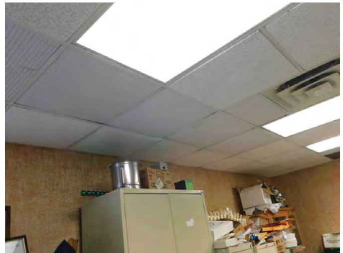
R5: CEILING FINISHES, CEILING TILE REPLACEMENT & ITEMS ABOVE FLOOR, DUE TO WATER INFILTRATION, RM 103, LEAK OCCURED RIGHT BEFORE OUR ARRIVAL, Photo 835
