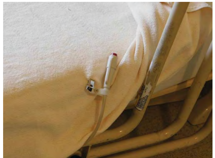
R8: NURSE CALL STATION, INOPERABLE & NEEDS TO BE REPLACED WITH ANTI-LIGATURE, Photo 1468
