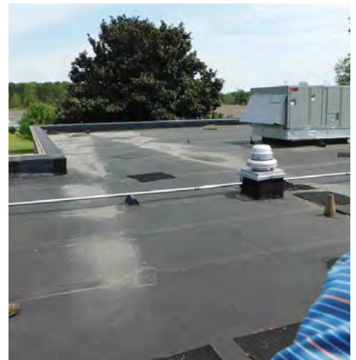
R3: LOW SLOPE MEMBRANE SYSTEMS, VIEW TO EAST, EVIDENCE OF PONDING, ABOVE ROOF LEAKS Photo 784
