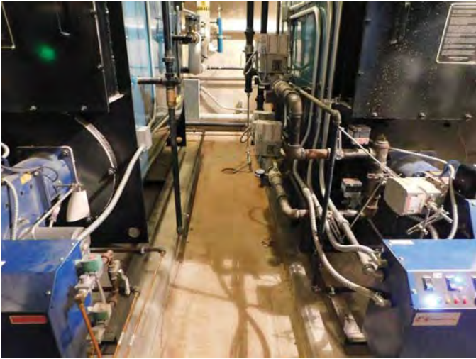
R6a: BOILER DRAIN FOR FLUSHING, RM B15, SEDIMENT ON FLOOR DUE TO FLOODING, Photo 1212
