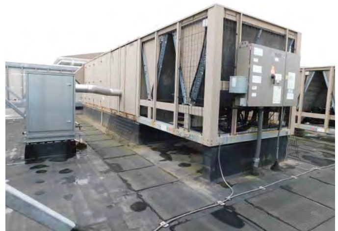
R3: HOSE BIB WOULD BE ADJACENT TO AHU'S. HOSE BIB NEEDED TO CLEAN ADJACENT COILS PERIODICALLY, Photo 1563
