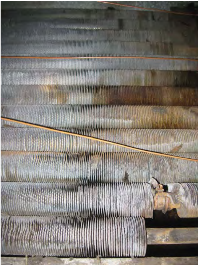
R12: BASEMENT H&V UNIT COILS, H-4 Photo 164
