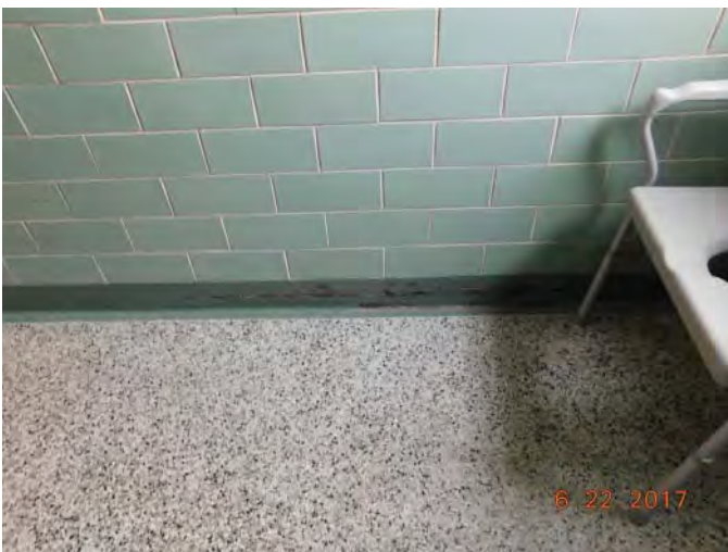
R7: CERAMIC TILE BASE CRACKED, RM 405 Photo 385
