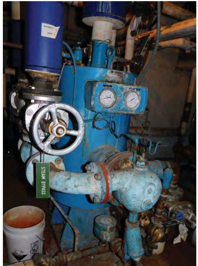
R14: REPLACE HEAT EXCHANGERS, NORTH AND EAST, Photo 44
