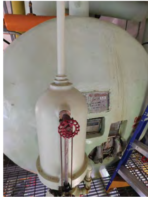
R13: DEAREATOR TANK, REPLACE, Photo SW 6012
