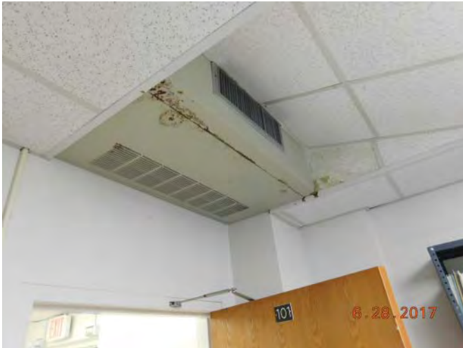
R16: FAN COIL UNITS NEED REPLACEMENT, RM 101, Photo 822
