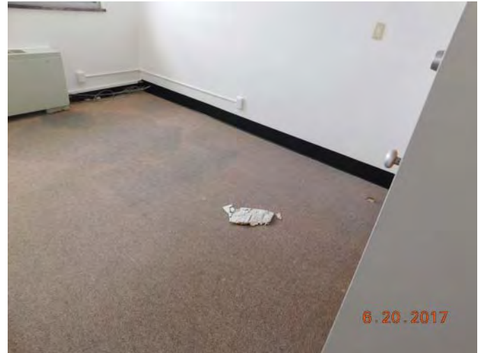
R6: CARPET STAINS, 8TH FLOOR, ROOMS, Photo 49
