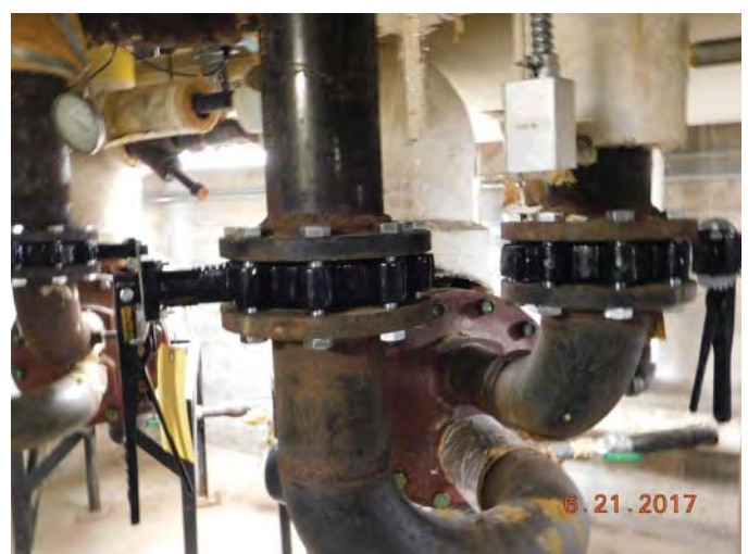
R12: REPLACE HEAT EXCHANGERS (TWO) BEYOND. SHELL NEEDS TO BE REPLACED. TUBES HAVE BEEN REPLACED. Photo 221
