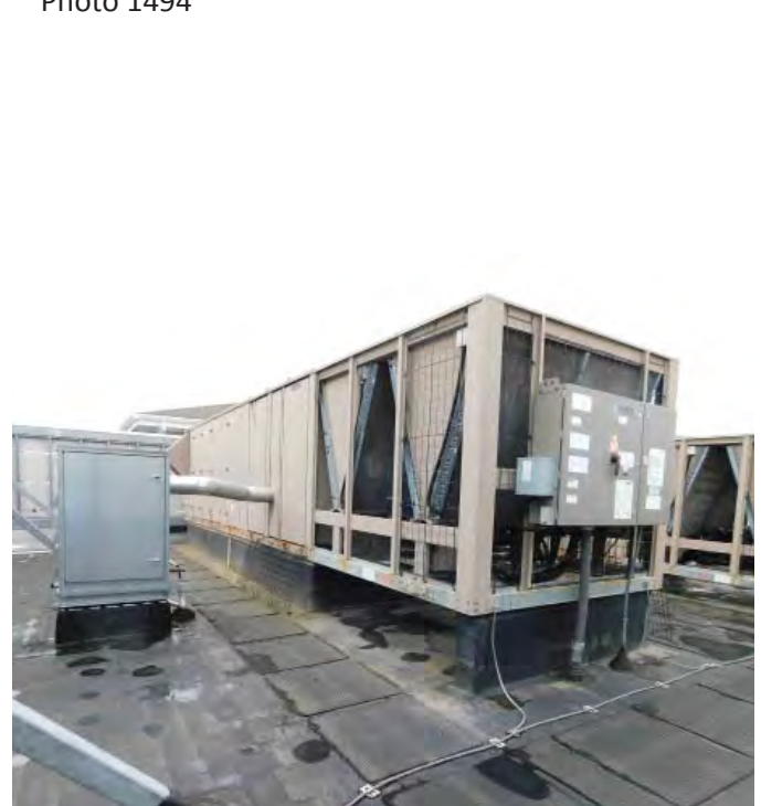
R3: HOSE BIB WOULD BE ADJACENT TO AHU'S. HOSE BIB NEEDED TO CLEAN ADJACENT COILS PERIODICALLY, Photo 1563
