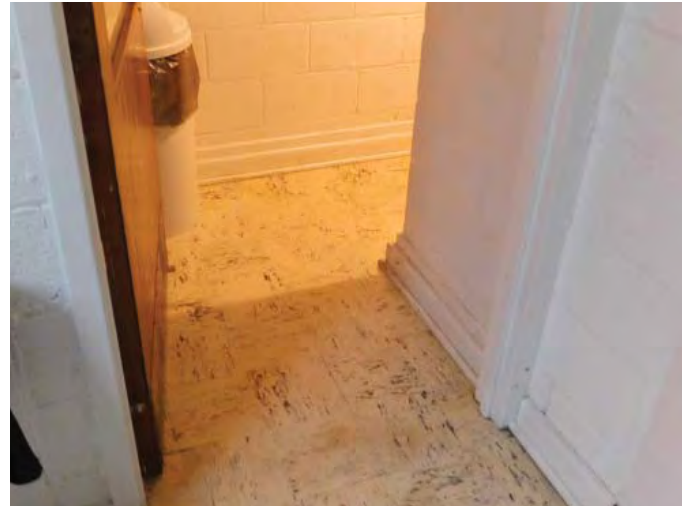
R27: REPLACE 9X9 ASBESTOS FLOOR TILES IN NORTH WING ROOMS G-75, G-74, AND STAIR 5, Photo 116
