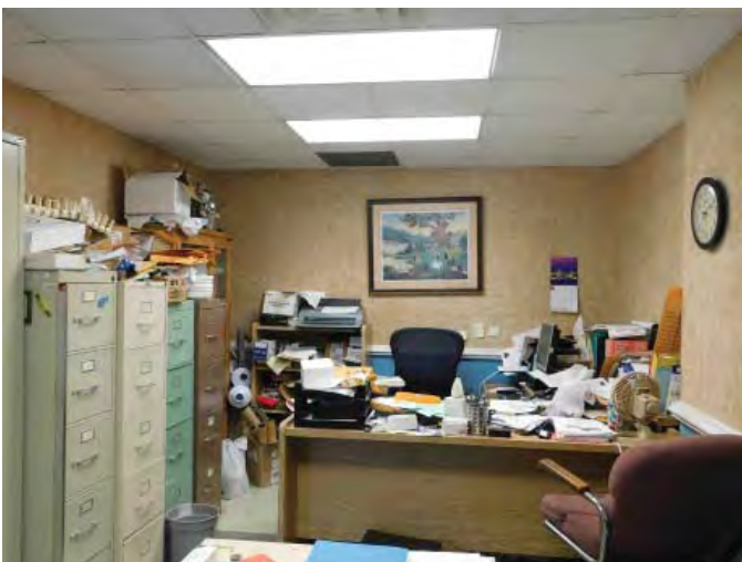
R5: CEILING FINISHES, CEILING TILE REPLACEMENT & ITEMS ABOVE FLOOR, DUE TO WATER INFILTRATION, RM 103, BUCKET ON FLOOR TO CATCH WATER, Photo 836
