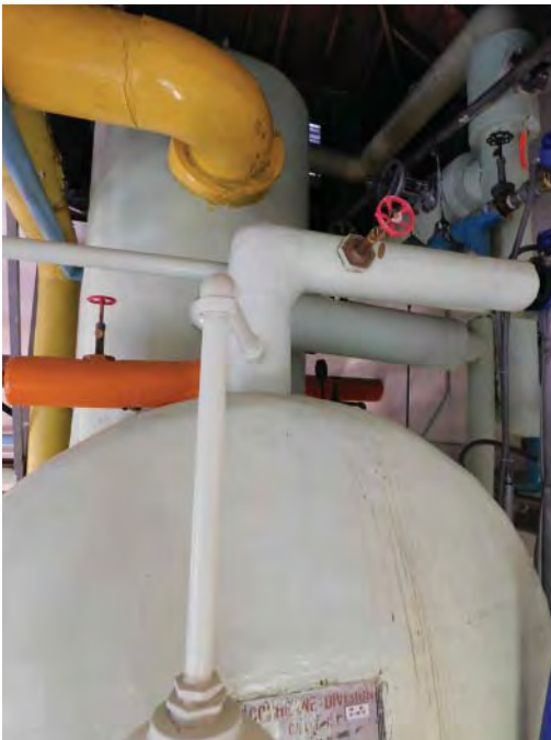
R13: DEAREATOR (DA) TANK REPLACE, Photo SW 6010
