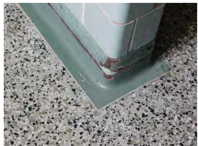
R7: CERAMIC TILE BASE CRACKED, RM 405, Photo 2396
