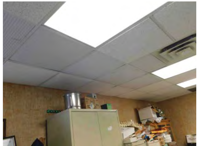
R5: CEILING FINISHES, CEILING TILE REPLACEMENT & ITEMS ABOVE FLOOR, DUE TO WATER INFILTRATION, RM 103, LEAK OCCURED RIGHT BEFORE OUR ARRIVAL, Photo 835
