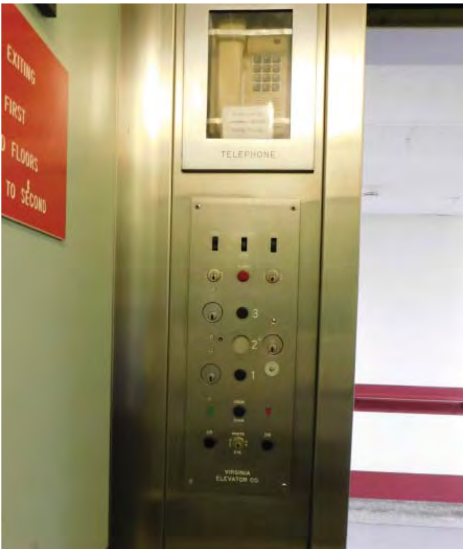
R9: PASSENGER ELEVATOR #3, Photo 65
