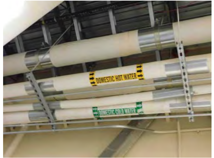
R4 SAGGING CVPC PIPING
