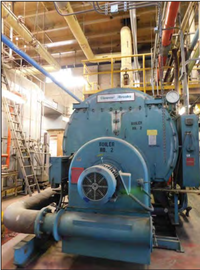
R21: STEAM BOILER, REPLACE BOILER #3, Photo 425
