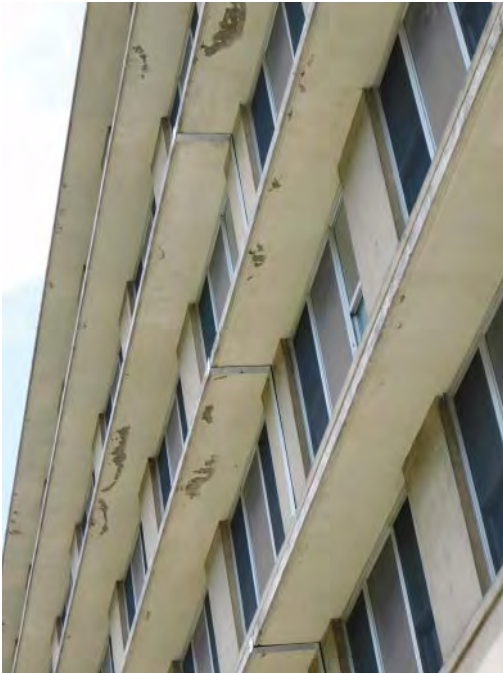
R3: EYEBROW (SOLAR SHADE) SPALLING AND LOOSE PAINT, SOUTH ELEV, Photo 1444
