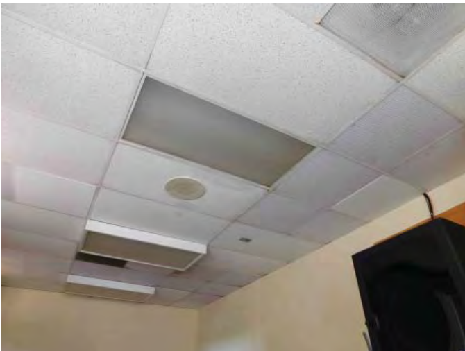
R5: CEILING FINISHES, CEILING TILE REPLACEMENT DUE TO WATER INFILTRATION, RM 103A, LEAK ABV AUDIO VISUAL EQUIPMENT, Photo 1158
