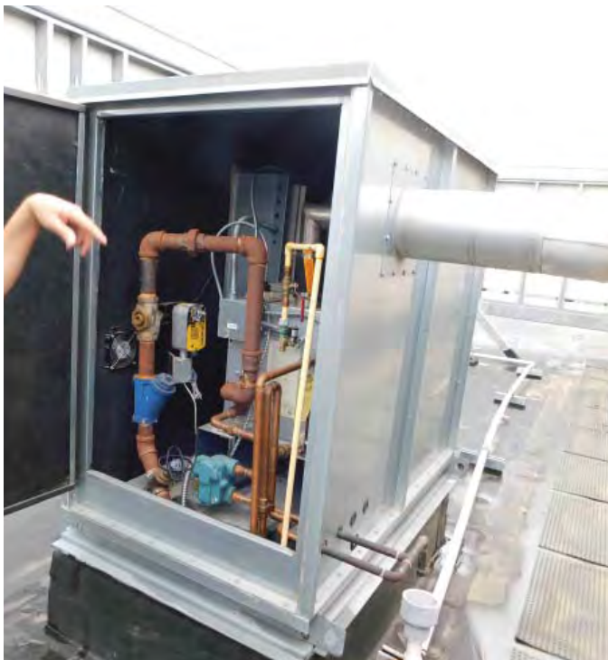
R3: REMOVE HUMIDIFIER NO LONGER IN USE. INSTALL HOSE BIB USING EXISTING PIPING, Photo 1560
