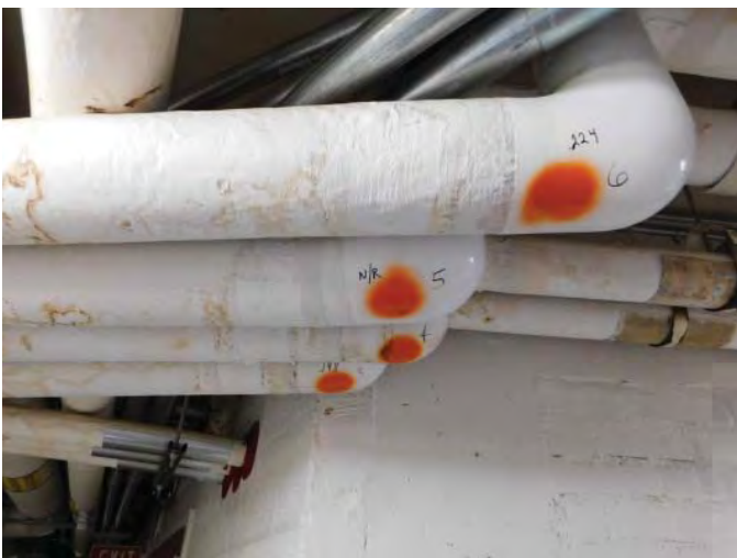
R16: DUAL TEMP PIPES Photo 167, RM B7
