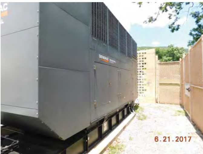
R19: ADD EMERGENCY POWER SWITCH TO BLDGS 17 & 23. Photo 257
