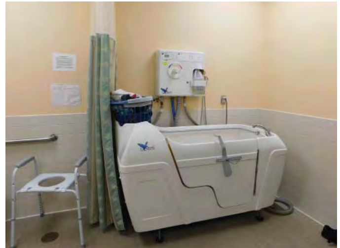
R2: LIBERTI TUB. ALL BATHTUBS LEAK THROUGH THE DOOR CLOSURE SEAL. Photo 1489
