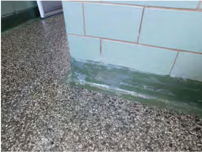
R7: CRACKED BASE TILE, RM 703 MEN'S Photo 3253
