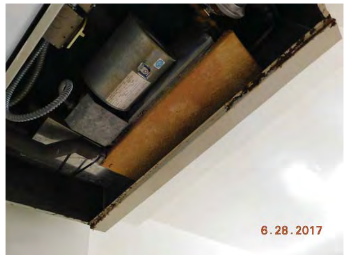
R16: FAN COIL UNIT CABINET REPLACE, Photo 788
