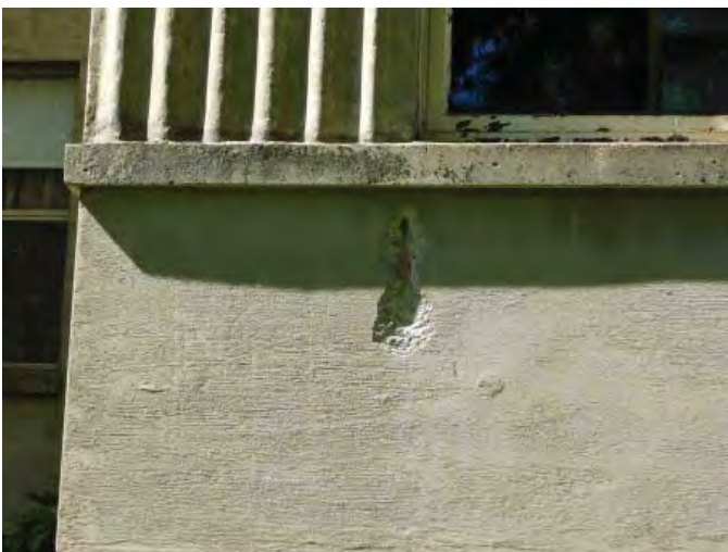
R2B: EXTERIOR WALL, SPALLING SELECT AREAS, EAST WING, SOUTH SIDE, Photo 716
