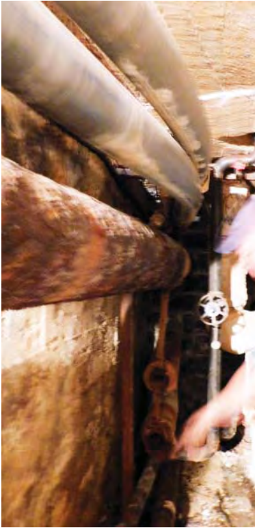
R12+ R12A: STEAM DISTRIBUTION LINES- CONDENSATE REPLACE, Photo SW 6052
