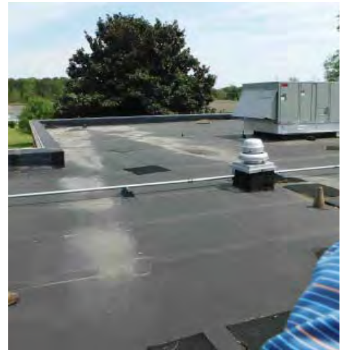
R3: LOW SLOPE MEMBRANE SYSTEMS, VIEW TO EAST, EVIDENCE OF PONDING, ABOVE ROOF LEAKS Photo 784
