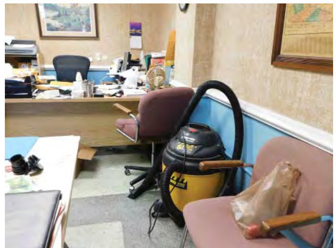
R5: CEILING FINISHES, CEILING TILE REPLACEMENT & SHOP VAC DUE TO WATER INFILTRATION, RM 103, LEAK OCCURRED RIGHT BEFORE OUR ARRIVAL, Photo 837
