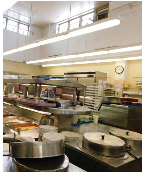
R14: EXHAUST SYSTEM FAN REPLACE, Photo SW 6936
