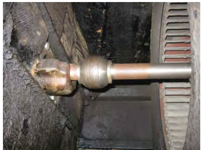
R12: BASEMENT H&V UNIT, H-4, COILS DAMAGED, BEYOND USEFUL LIFE, Photo 165
