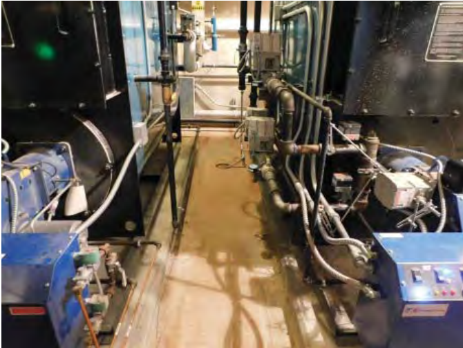
R6: BOILER NEW DRAIN NEEDED FOR FLUSHING. RM B15, SEDIMENT ON FLOOR DUE TO FLOODING, Photo 1212
