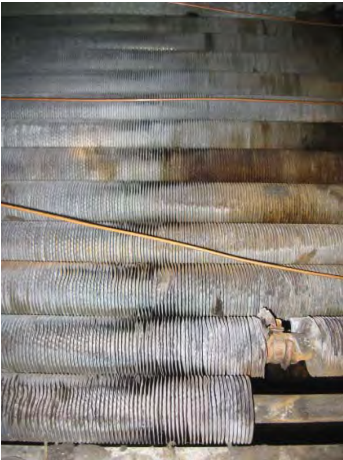
R12: BASEMENT H&V UNIT COILS, H-4 Photo 164
