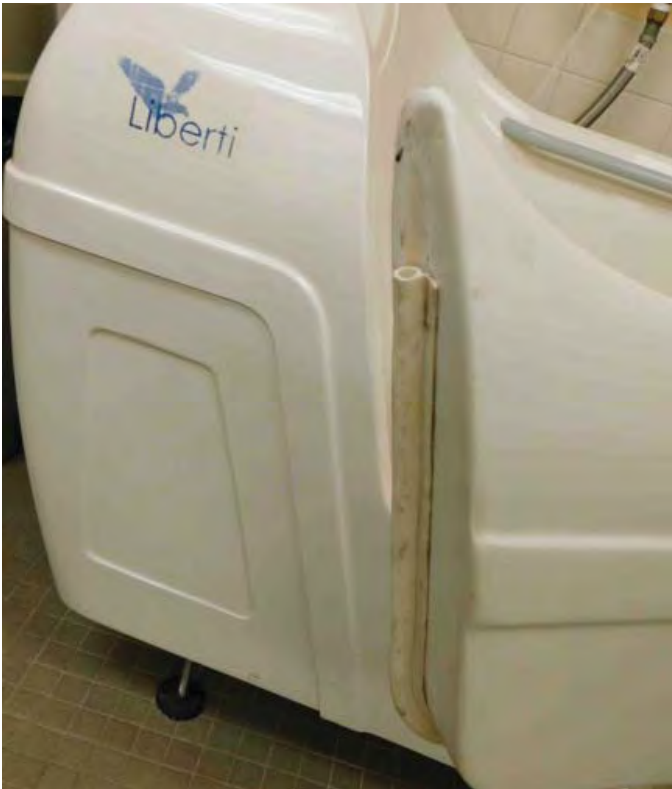
R2: LIBERTI TUB. TUBS LEAK THROUGH THE DOOR CLOSURE SEAL. Photo 2414
