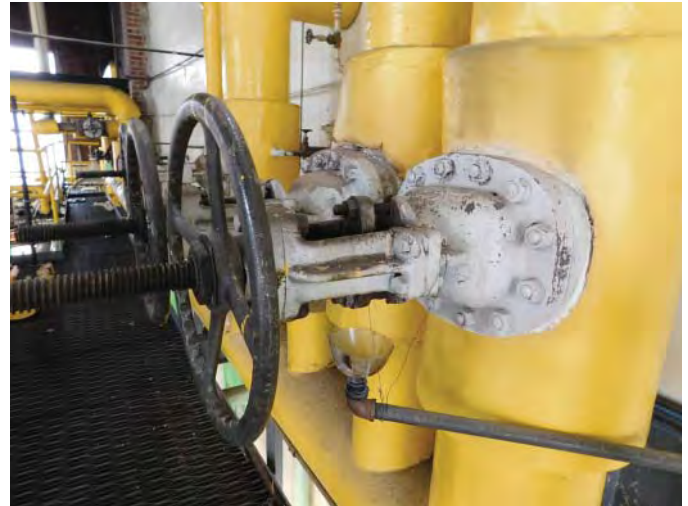
R9: DOMESTIC WATER DISTRIBUTION- VALVE HEADS 6" FLANGES REPLACE, Photo SW 5977
