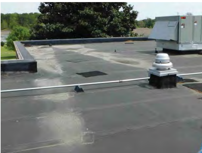
R3: LOW SLOPE MEMBRANE SYSTEMS, VIEW TO EAST, EVIDENCE OF PONDING WATER, Photo 784
