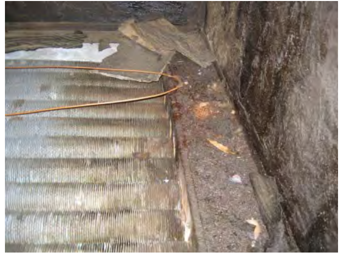
R12: BASEMENT H&V UNIT, H-4, COILS DAMAGED, BEYOND USEFUL LIFE,
