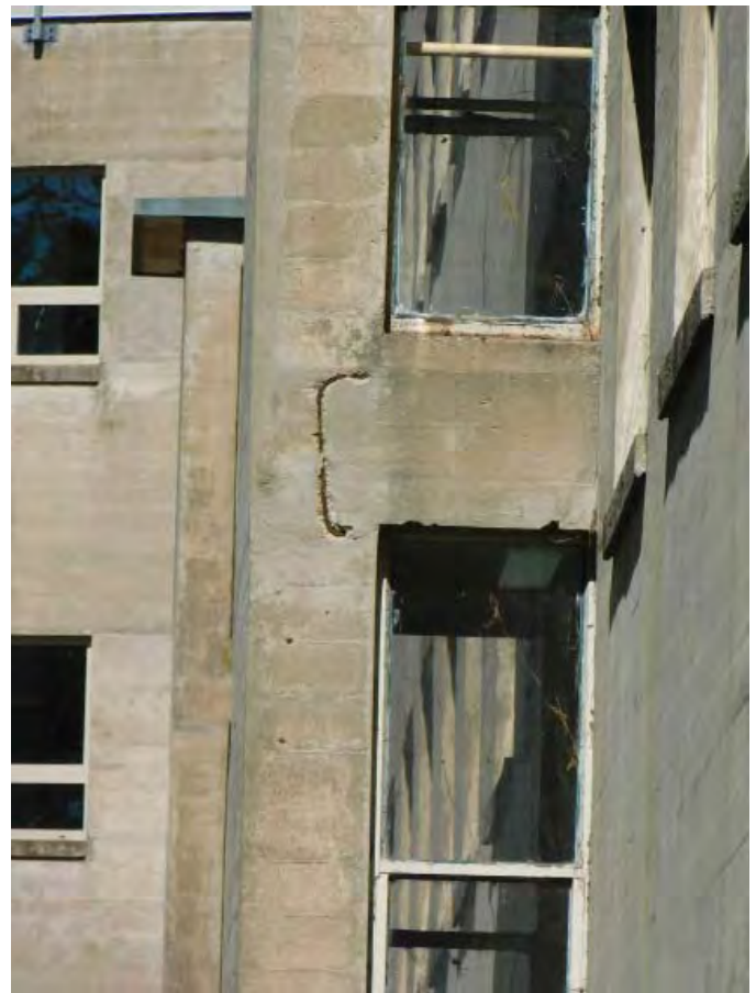
R2B: EXTERIOR WALL, SPALLING SELECTED AREAS, WEST WING, NORTH SIDE Photo 646
