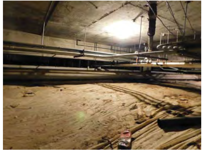
R11: SANITARY WASTE PIPING IN CRAWL SPACE, Photo 850
