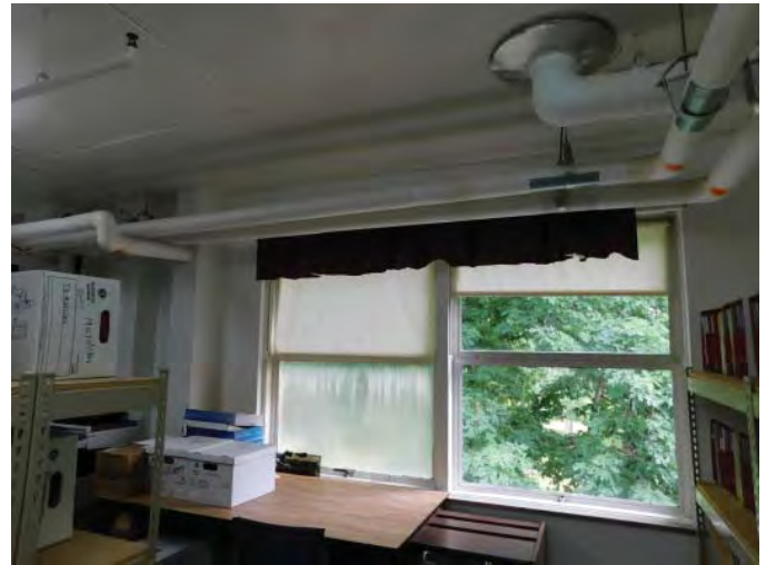
R10: EAST WING DOMESTIC PLUMBING PIPES, Photo 562, Rm 371
