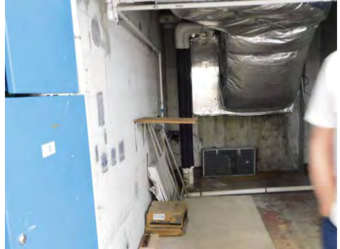
R13: RM G68 ADD DRAIN FOR AHU-5 Photo 396
