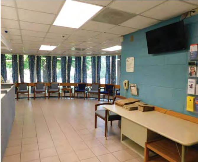
R8: PUBLIC ADDRESS SYSTEM-REPLACE, Photo SW 4933
