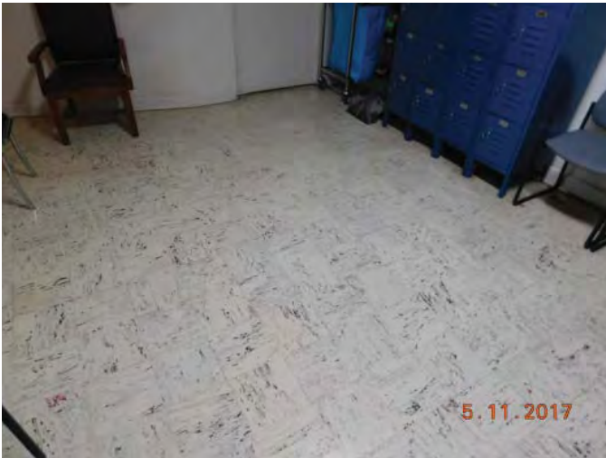
R27: REPLACE 9X9 ASBESTOS FLOOR TILES IN NORTH WING ROOMS G-75, G-74, AND STAIR 5, Photo 114
