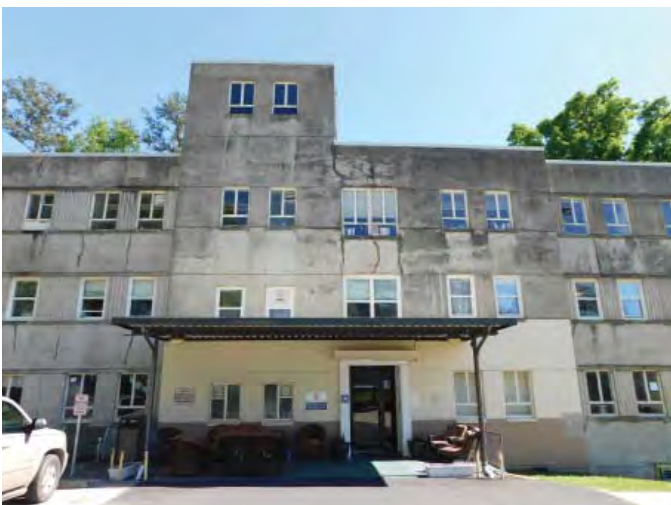
R4: WINDOWS, EAST WING NORTH ELEV Photo 756
