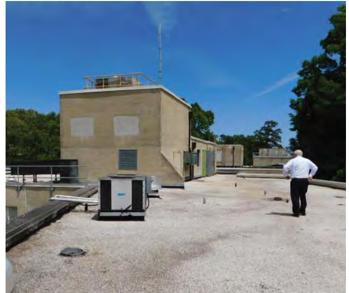
R1: PARAPET, RAILING NEEDED AT BLDG OFFSET, Photo 65
