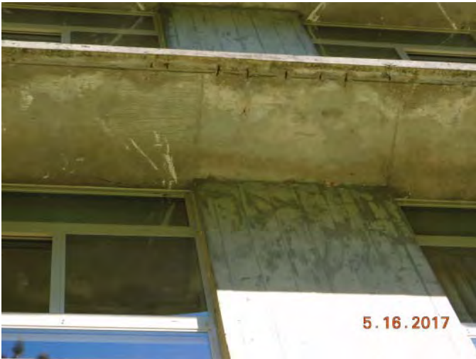
R2C: CONCRETE SHADE, WEST WING, SOUTH SIDE, SPALLING, Photo 520
