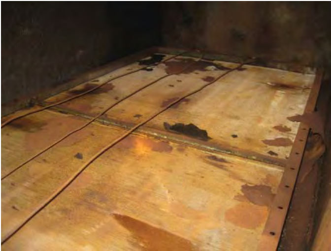
R12: BASEMENT H&V UNIT, H-4, COILS DAMAGED, BEYOND USEFUL LIFE, Photo 172
