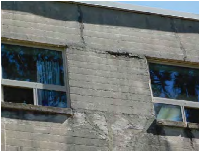
R2B: EXTERIOR WALL, SPALLING SELECTED AREAS, WEST WING, NORTH SIDE Photo 653
