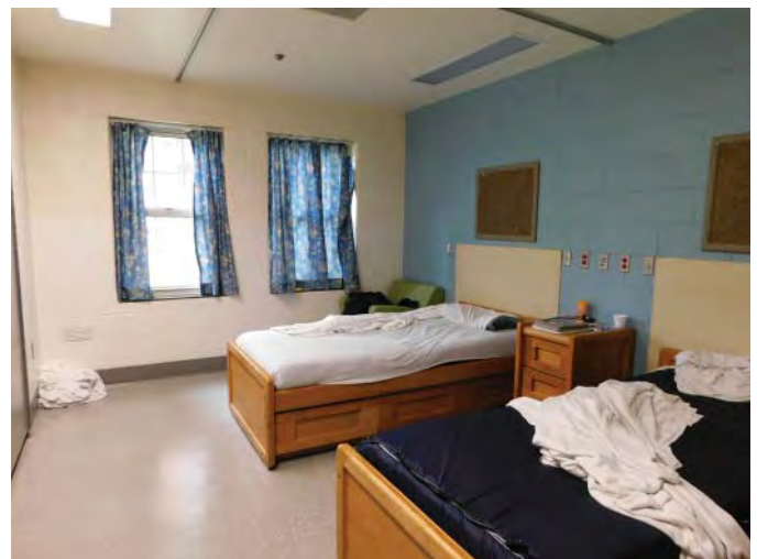
R2A: FLOOR FINISHES, PATIENT CORRIDORS & ROOMS REPLACE, RM D-104, Photo 6310
