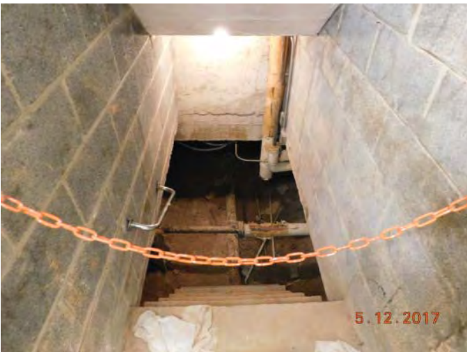
R13A: PIPE IN CRAWL SPACE , STR 4 Photo 221
