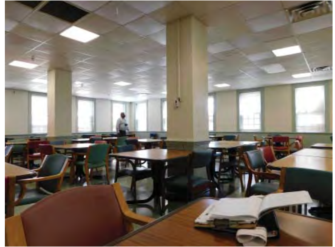
R5: CEILING FINISHES, CEILING TILE REPLACEMENT DUE TO WATER INFILTRATION, RM 102, Photo 731
