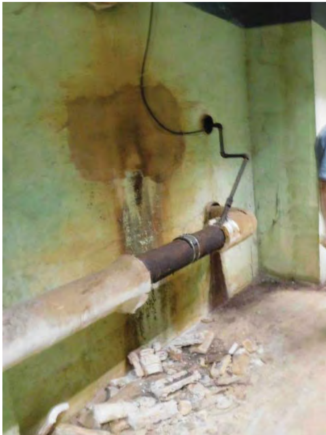
R13 & R14: STEAM & CONDENSATE PIPING, CORRODED PIPE & MISSING INSULATION, Photo 872
