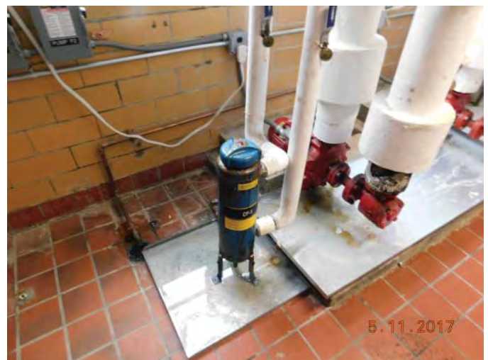
R20: RM G-71 NEEDS EVAPORATION UNIT
