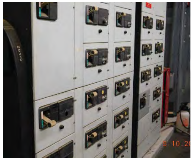
R23: MOTOR CONTROL CENTER Photo 16
