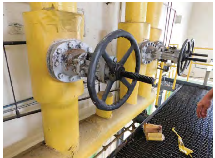
R11: DOMESTIC WATER DISTRIBUTION- VALVE HEADS 8" SAFETY VALVES REPLACE, Photo SW 5983
