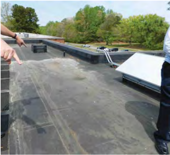
R3: LOW SLOPE MEMBRANE SYSTEMS, VIEW TO NORTH, EVIDENCE OF PONDING, (ABV RM 103 CEILING LEAKS) Photo 776
