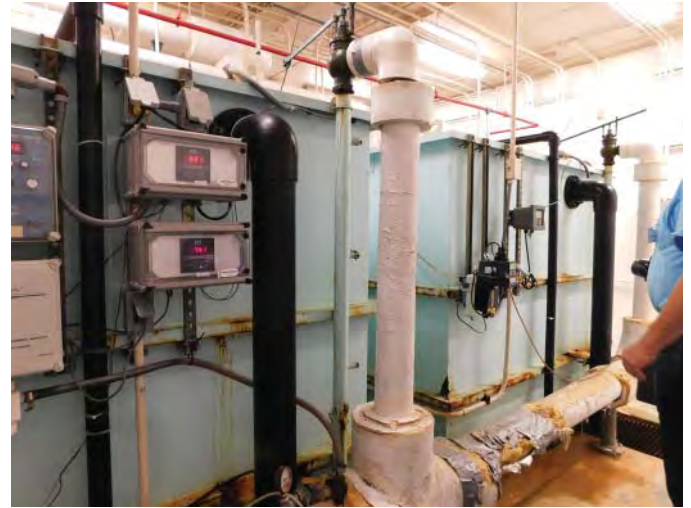
R20: REPLACE WATER TREATMENT PLANT FILTRATION TANKS, Photo 2017
