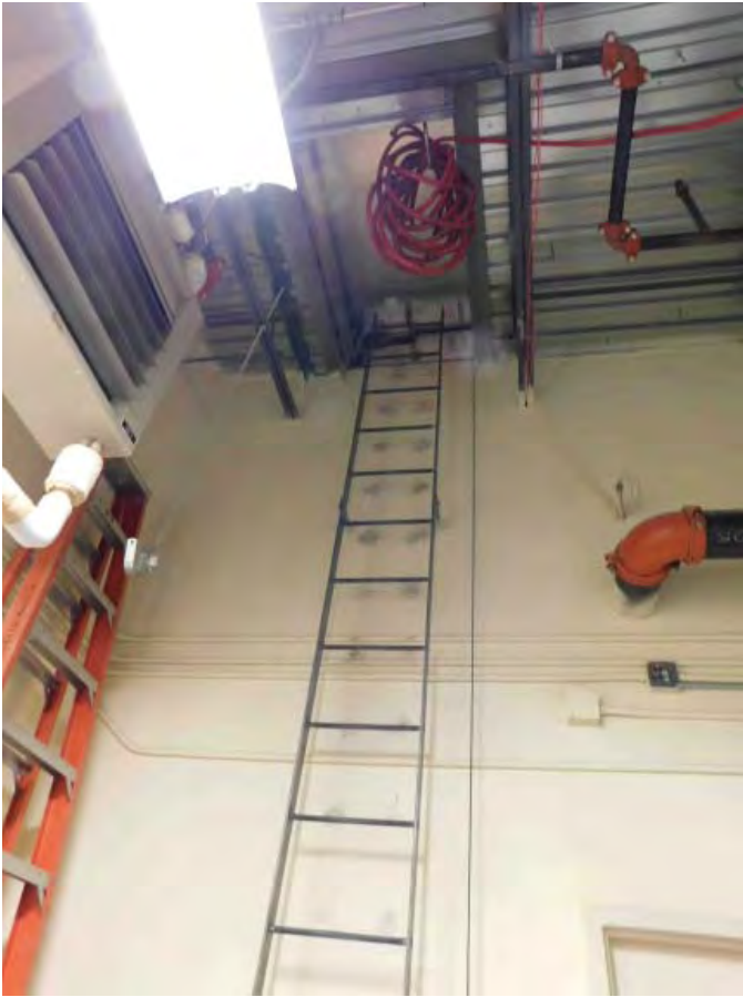
R1: SHIP'S LADDER, NO FLAT TREADS, HANDRAILS OR SAFETY CAGE, DIFFICULT TO CLIMB W/ EQUIPEMENT, Photo 1401
