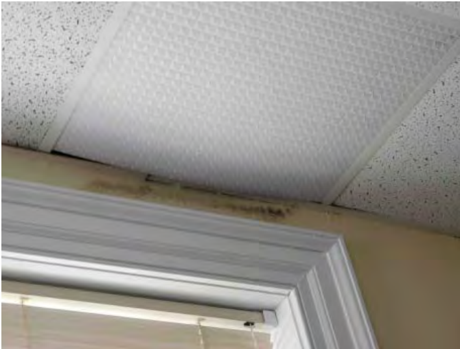
R5: CEILING FINISHES, CEILING TILE REPLACEMENT & WATER STAIN, DUE TO WATER INFILTRATION ABOVE WINDOW, RM 103A, Photo 744
