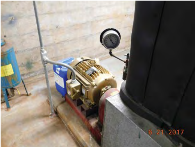
R17: DDC / PNEUMATIC SYSTEM HYBRID RENEWAL, Photo 227
