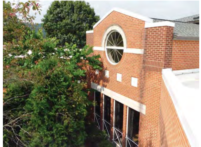
R1: EXTERIOR WINDOWS , Photo SW 5568
