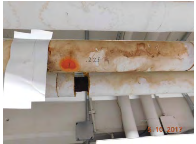
R16: DUAL TEMPERATURE PIPES Photo 49c, RM B7
