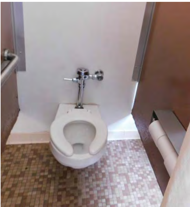
R5: REPLACE PARTITION AS RUSTED, Photo 103
