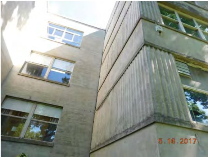
R1: PARAPET, RAILING NEEDED AT BLDG OFFSET, Photo 544 c
