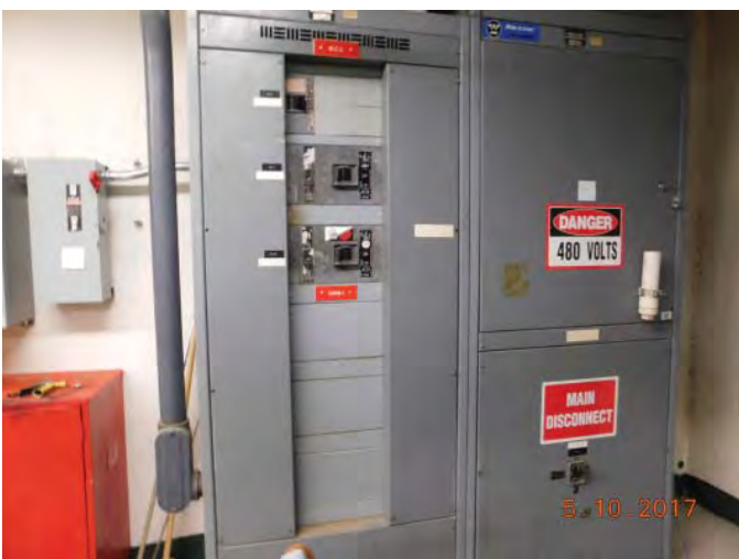
R22: TRANSFER SWITCH Photo 13
