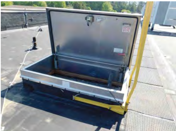
R1: TOP OF SHIP'S LADDER. LACK OF HANDRAIL AT TOP, Photo 1578d
