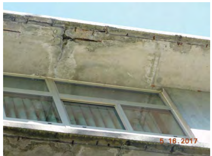
R2C: CONCRETE SHADE, WEST WING, SOUTH SIDE, SPALLING, Photo 530
