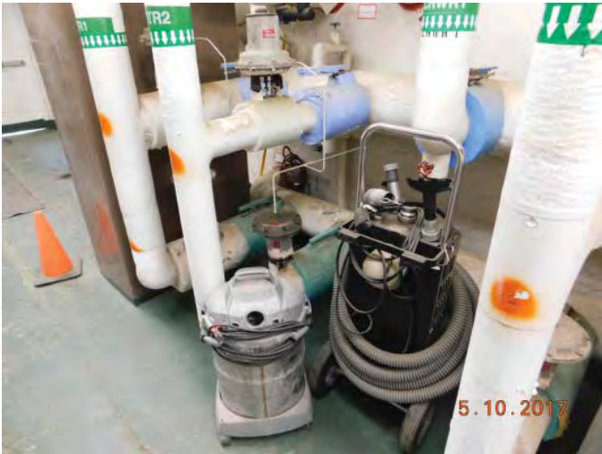
R15: CHILLER ROOM PIPING AND COOLING TOWER, Photo 4
