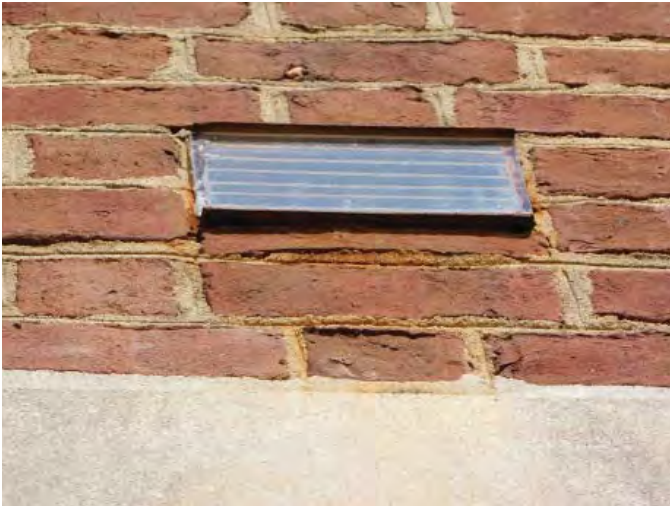
R1: BRICK VENT, WITH PLASTIC COVER, NOT ALLOWING VENTILATION Photo 897
