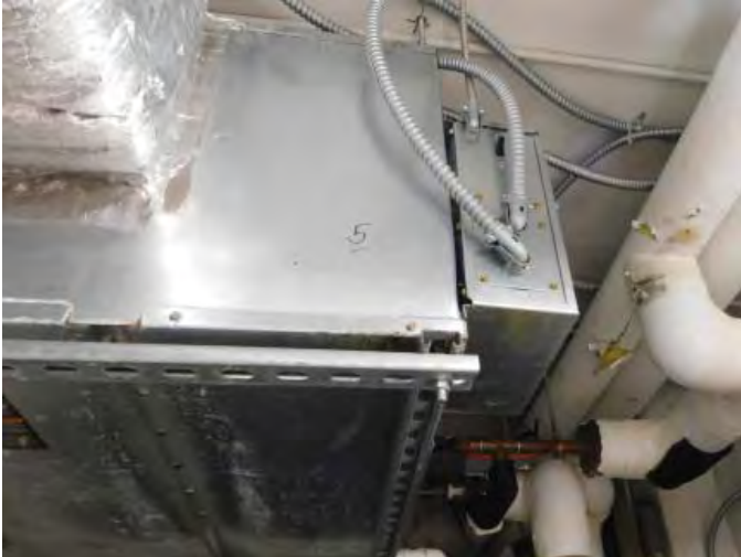
R13: RM G68 ADD DRAIN FOR AHU-5 Photo 399
