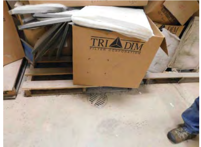
R6: BOILER NEW DRAIN NEEDED FOR FLUSHING. N-S CORRIDOR DRAIN, ELEVATED BOXES & SEDIMENT ON FLOOR DUE TO FLOODING, Photo 1212
