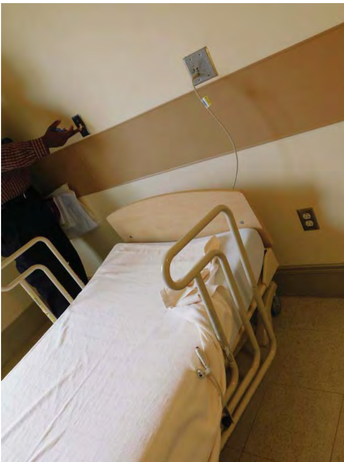
R7: NURSE CALL STATION, INOPERABLE & NEEDS TO BE REPLACED WITH ANTI-LIGATURE, Photo 1467
