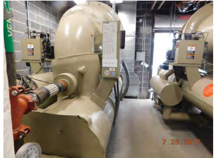
R4-5: DISTRIBUTION SYSTEMS-CHILLED WATER, LINES TO BE SPLIT, INSULATE LINE, Photo SW 262
