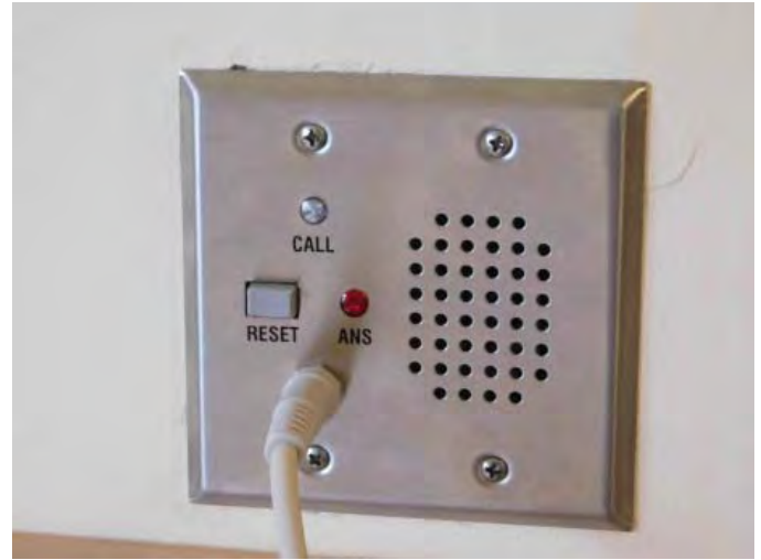
R7: NURSE CALL STATION, INOPERABLE & NEEDS TO BE REPLACED WITH ANTI-LIGATURE, Photo 1466
