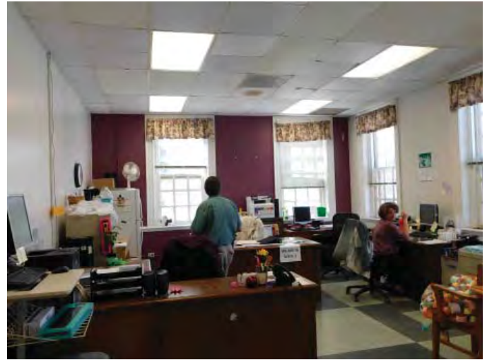
R5: CEILING FINISHES, RM 101A, REPLACEMENT CEILING TILES DUE TO WATER INFILTRATION, Photo 823
