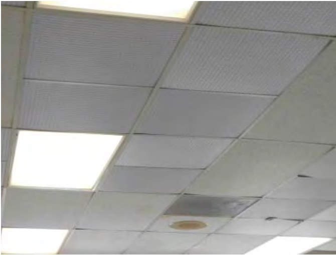
R5: CEILING FINISHES, RM 101A, REPLACEMENT CEILING TILES DUE TO WATER INFILTRATION, Photo 822
