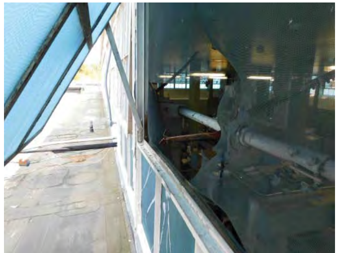
R2 & 2A: REPLACE STEEL WINDOWS & SCREENS, WINDOW FRAME BENT, OPERATOR ARM DETACHED, SCREEN RIPPED Photo 810
