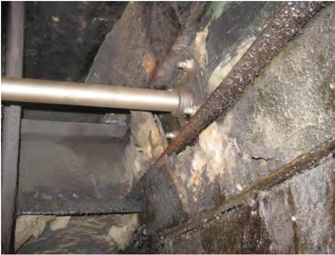
R12: BASEMENT H&V UNIT, H-4, COILS DAMAGED, BEYOND USEFUL LIFE,
