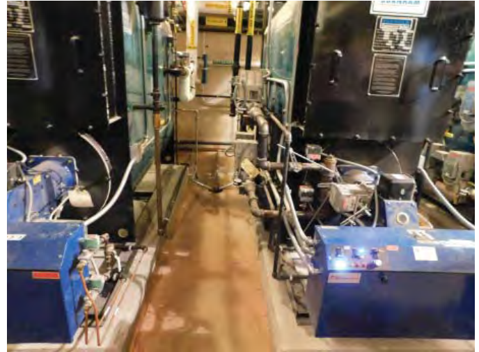
R6: BOILER NEW DRAIN NEEDED FOR FLUSHING. SEDIMENT ON FLOOR DUE TO FLOODING, Photo 1211
