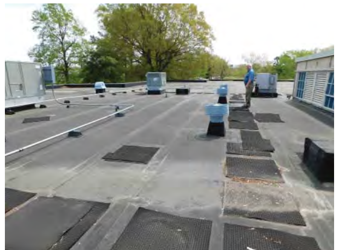
R3: LOW SLOPE MEMBRANE SYSTEMS, VIEW TO NORTH, EVIDENCE OF PONDING, Photo 785
