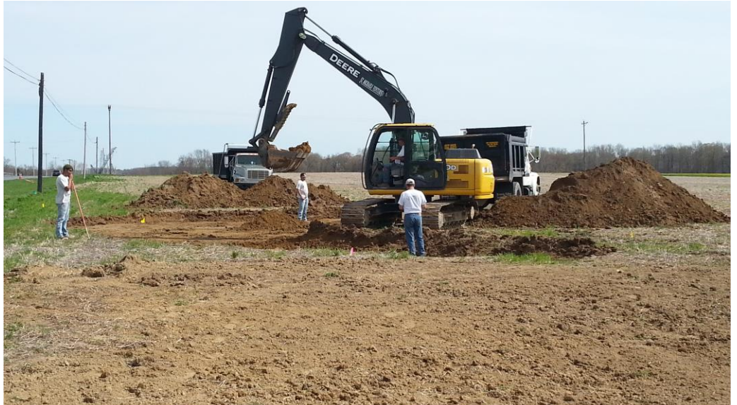
Construction of wetland cells/ detention basins at the upper end of grass waterway at the Dover Road Site.
