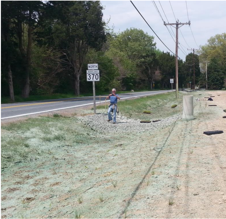
Unionville Road site post-restoration April 2016. The site was hydro-seeded and planted with wetland plants. Alan Girard is standing on one of the rock weirs designed to slow the flow of water and increase nutrient retention.
