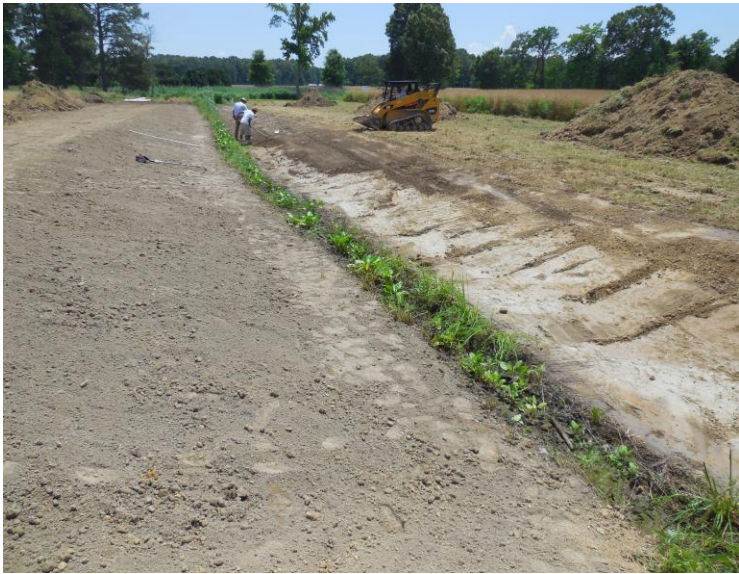
Bellevue Field Ditch during construction, creating wetland benches on both sides of ditch to improve water quality, June 2016.
