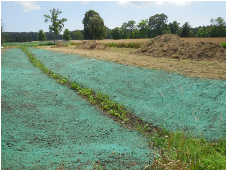
Bellevue Field Ditch during construction, after top soil and seeding, the area was hydro-mulched as an alternative stabilization technique that avoid the use of matting that may contain plastic, June 2016.
