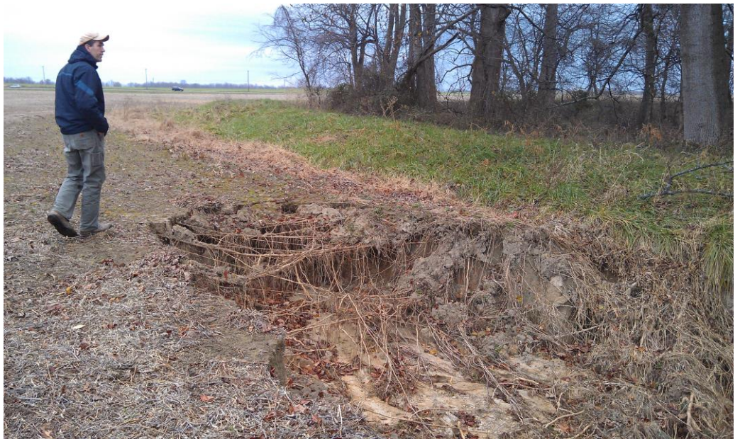
Erosion issue at the edge of farmfield leading into a headwater stream on the Dover Road site. The project addressed both water quality and erosion concerns.
