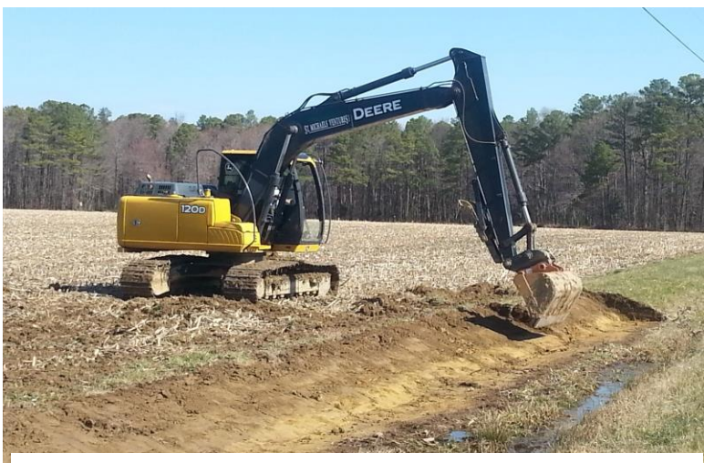
Bellevue Road 2-stage roadside ditch during construction in March 2015. A 5ft. wetland bench was created on the field side of the ditch.
