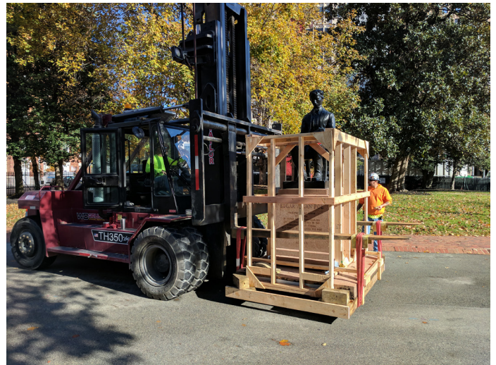
Fine Art Specialists moving the Poe Statue to its new location at the northwest corner of Capitol Square. Source: CSPC
