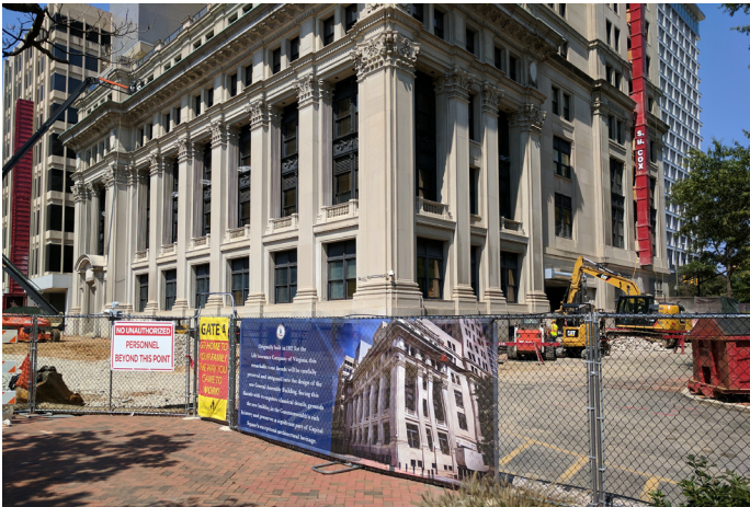
Initial demolition and abatement of the General Assembly Building, Fall 2017. Source: CSPC.
