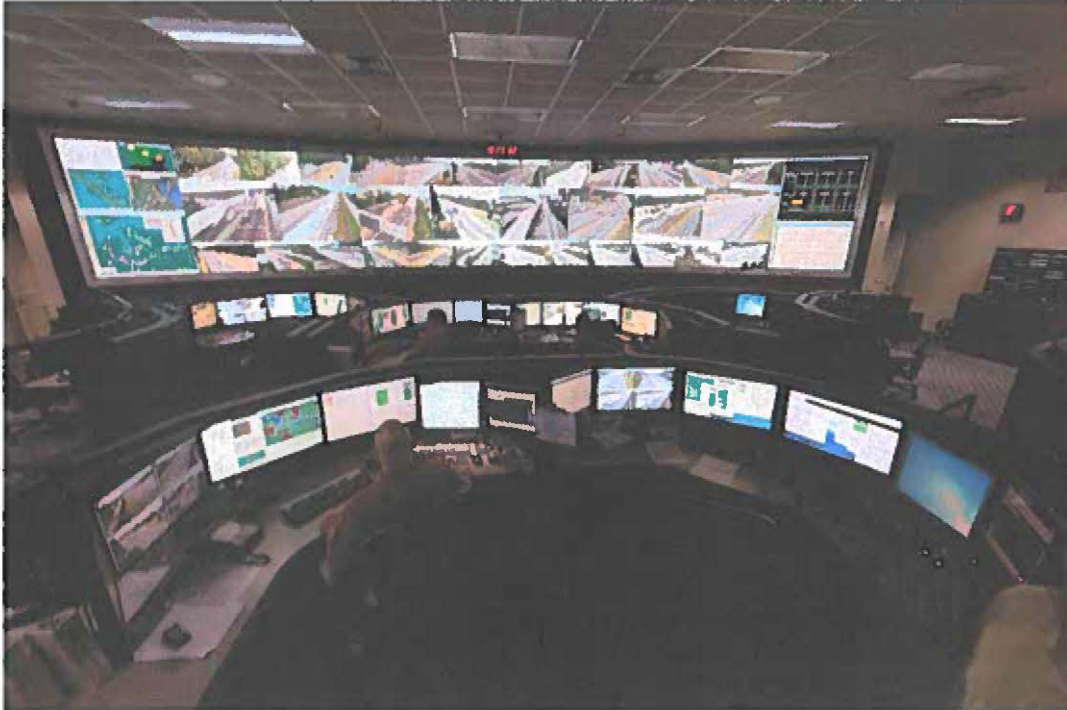
Figure 46: Traffic Operations Center – Hampton, VA
