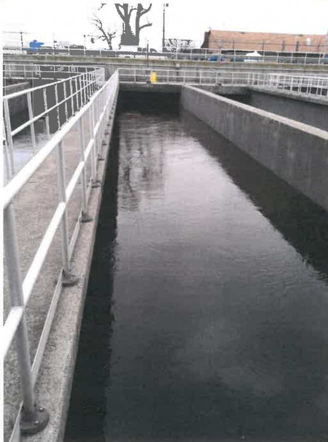
NEORSD Easterly Plant: Chlorine Contact Tank
