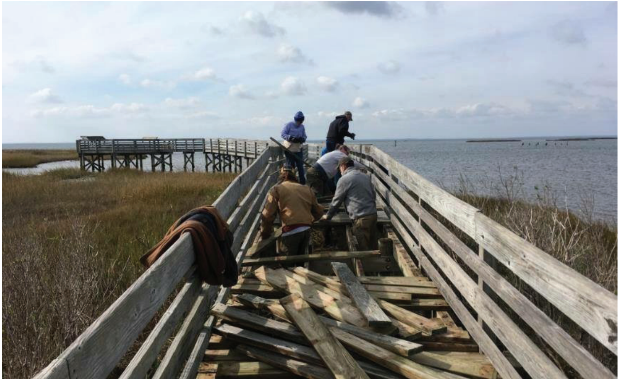
Local volunteers assist DCR stewards with repairs to the boardwalk at New Point Comfort Natural Area Preserve in Mathews County.
