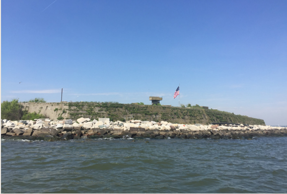
The view of Fort Wool's deteriorating sea wall.
