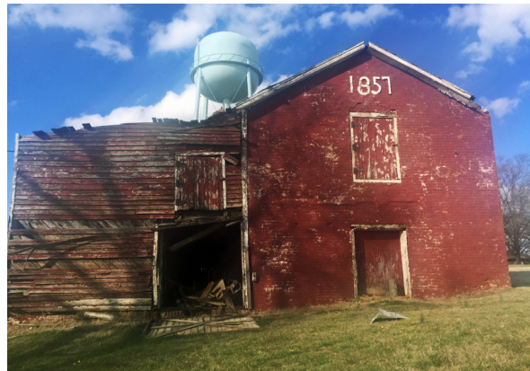
The Mule Barn at the former Powhatan Correctional Facility was demolished due to deterioration from neglect.
