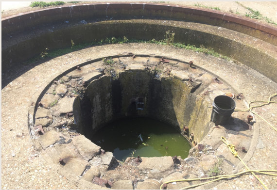
A plugged drain needing cleaning out.
