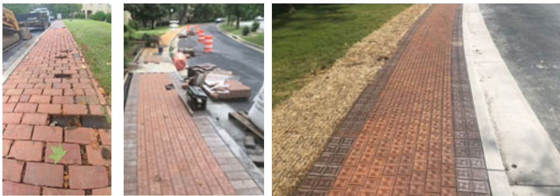
L-R: The brick walk at VMI prior to rehabilitation, during construction, and after completion.
