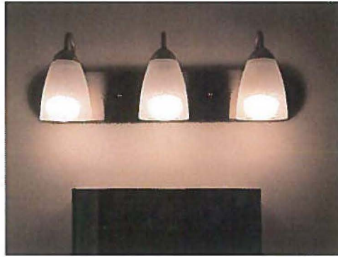
New LED lighting
