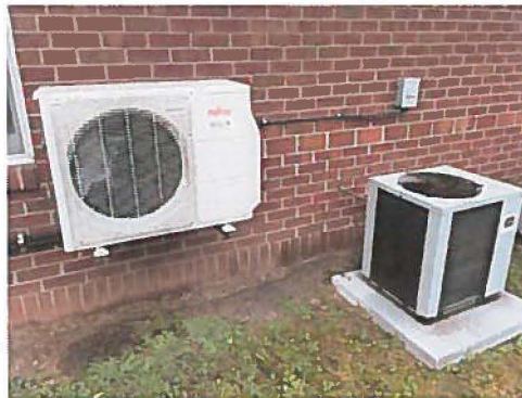
Photo of new mini-split heat pump (left) and the existing heat pump (right)
