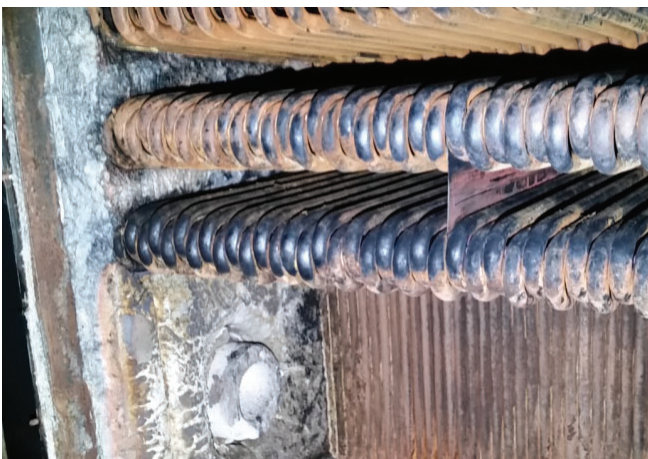
Watertube boiler (black pipes can be an indicator of scale buildup)
