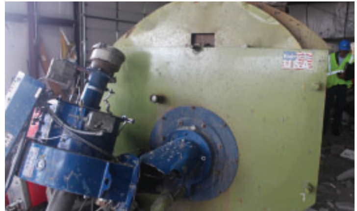
Detail of aftermath of boiler explosion (Petersburg, Virginia)
