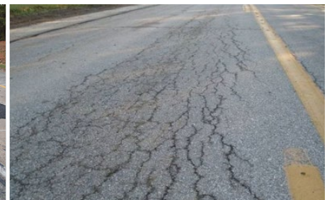
Poor to Very Poor Pavement
