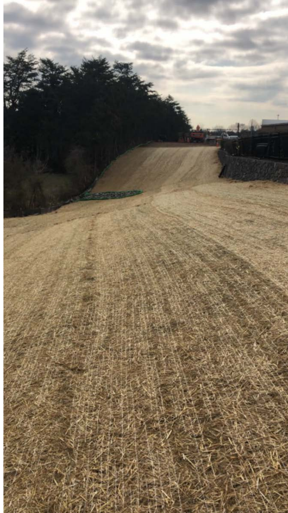
Western HDD Drill Path Drill Pad 4 (Kohl's Haymarket) Drill Pad 3 (Jordan Lane):
