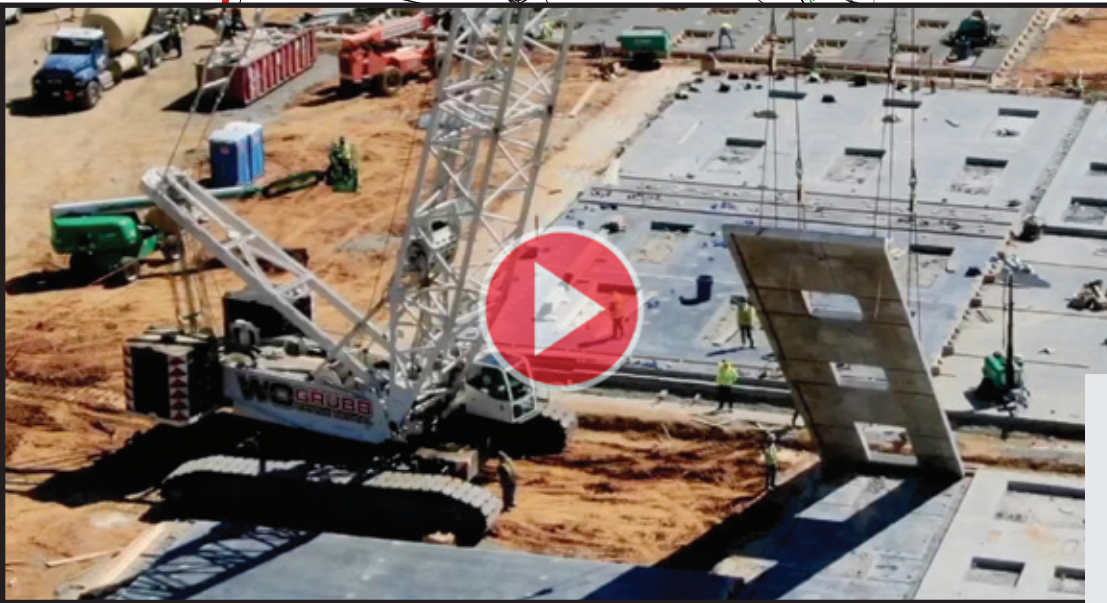
LEFT: With site preparation for ABC’s future headquarters and distribution center completed, footers and floors were poured before the first pre-cast concrete wall was hoisted into place on June 1, 2019. View the “First Wall” video at https://vimeo.com/virginiaabc .
