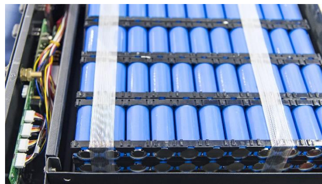
Figure 6. A lithium-ion battery module comprised of many individual cells. Large numbers of these cells put together form a large-scale lithium-ion deployment.
