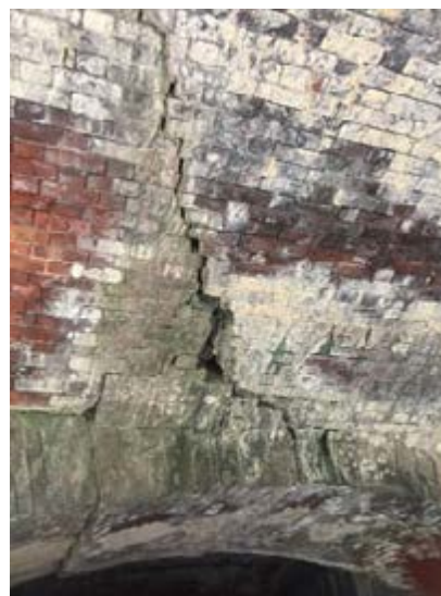
The casemate beginning to fail (2019).
