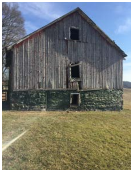
Barns at DOC properties photographed in 2017 show signs of deterioration.
