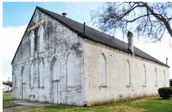
The registers-listed chapel building at CSH collapsed in 2014.
