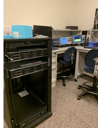
(c) Rack and bench in indoor testbed lab.
