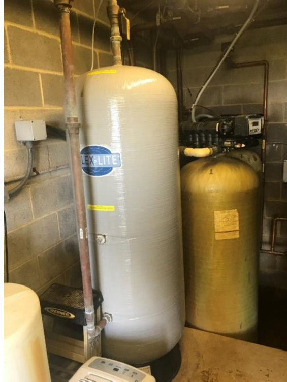
Photograph 3 – Iron & Manganese Treatment System
