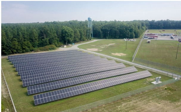
300 kilowatt solar installation at the Virginia Public Safety Training Center in Hanover County is one of several solar projects installed at Commonwealth facilities as part of Governor Northam's Lead-by-Example initiative
