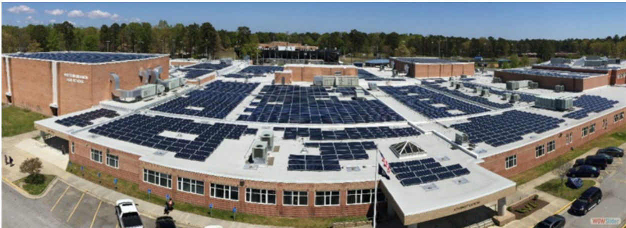
800 kilowatt solar installation at Western Branch High School in Chesapeake, Virginia Installed as part of Dominion Energy's Solar Partnership Program
