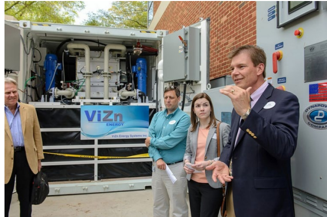
Dominion Resources installed solar coupled with a zinc iron redox flow battery made by Vizn Energy at Randolph Macon College in Ashland, Virginia as part of a microgrid test case.
