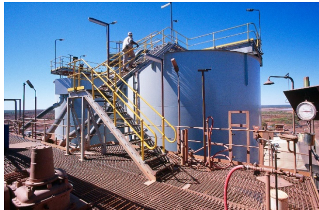
FIGURE 3-18 Cyanide leaching in tank at gold processing plant.
