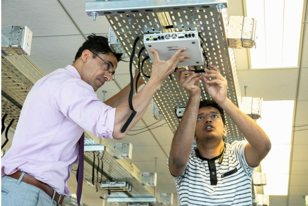
Figure 1.6: CCI xG Testbed Director Aloizio P. DaSilva (at left) installs 72 radio nodes in the Commonwealth Cyber Initiative test bed in Arlington with help from graduate student Vikas Radhakrishnan. The test bed was named one of 15 O-RAN testing and integration centers in the world and the only one in the greater Washington, D.C., metro area. Photo by Anthony Wright for Virginia Tech.
