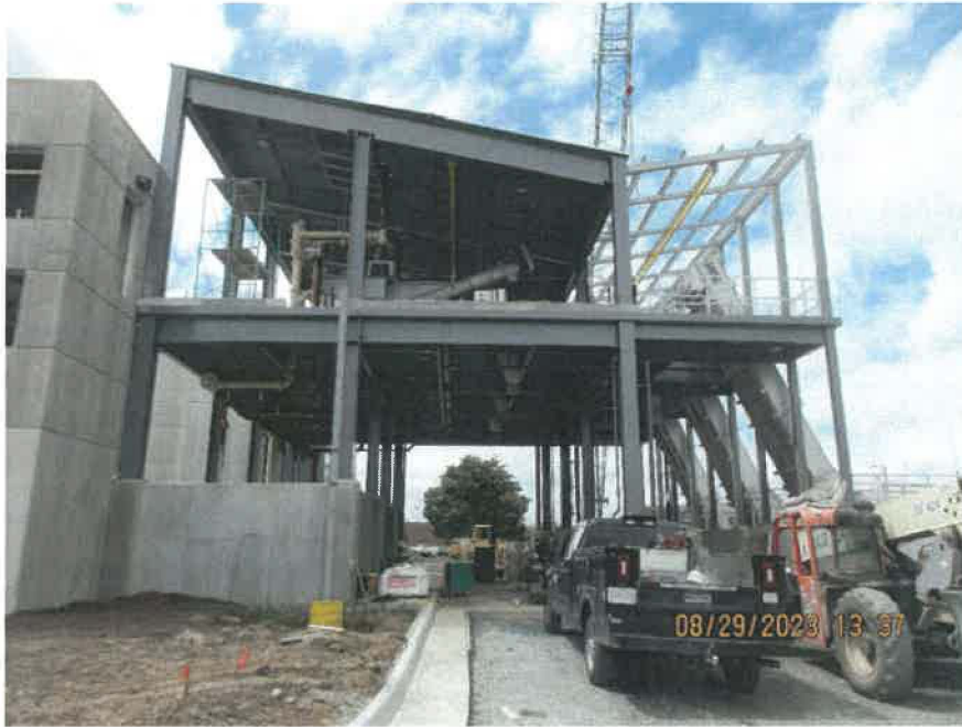
Construction of the Wastewater Treatment Plant's new Screening and Grit Building, which will remove harmful debris before entering the treatment facility, August 29, 2023.
