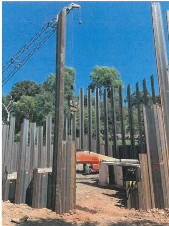
Construction of Outfall 004 Interim Plan Project will reduce annual overflow events at this location by 95%, August 1, 2023.
