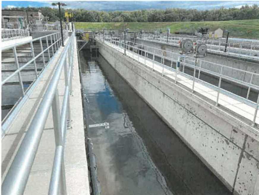
Figure 6. High-Rate Disinfection Facility Example
