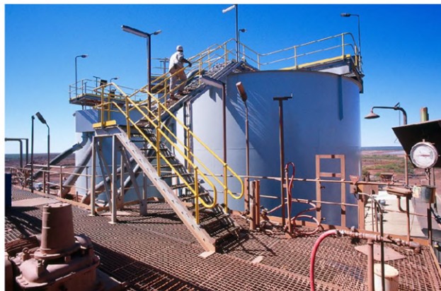
Gold processing tank
