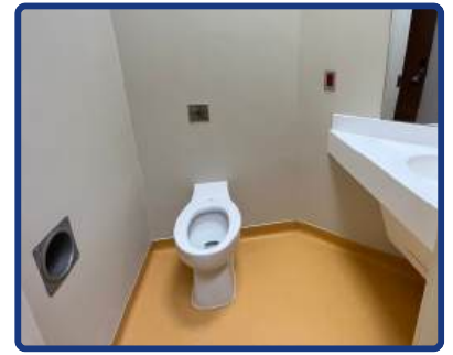
Absent grab bar for toilet in DBHDS facility.
